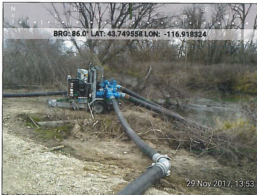
Figure 1: Two portable pumps diverting from the Boise River. Pump 1 with John Deere engine is further east, behind Pump 2 with Perkins engine.
