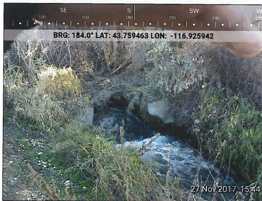
Figure 6: Boise River source water is piped under the Parma Ditch and returned to the Boise River.
