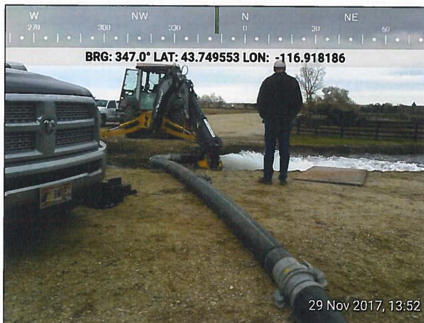
Figure 2: Pump 1 discharging into ditch and flowmeter installation.
