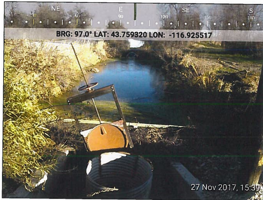
Figure 5: Lower end of Boise River source water collection ditch and entrance to pipeline under Parma Ditch.
