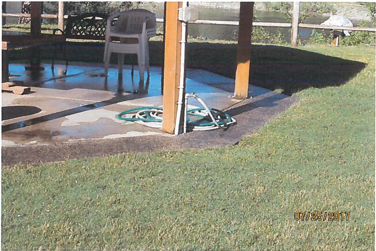
Frost free hydrant where 5 gallon bucket test was performed in 10 seconds.
