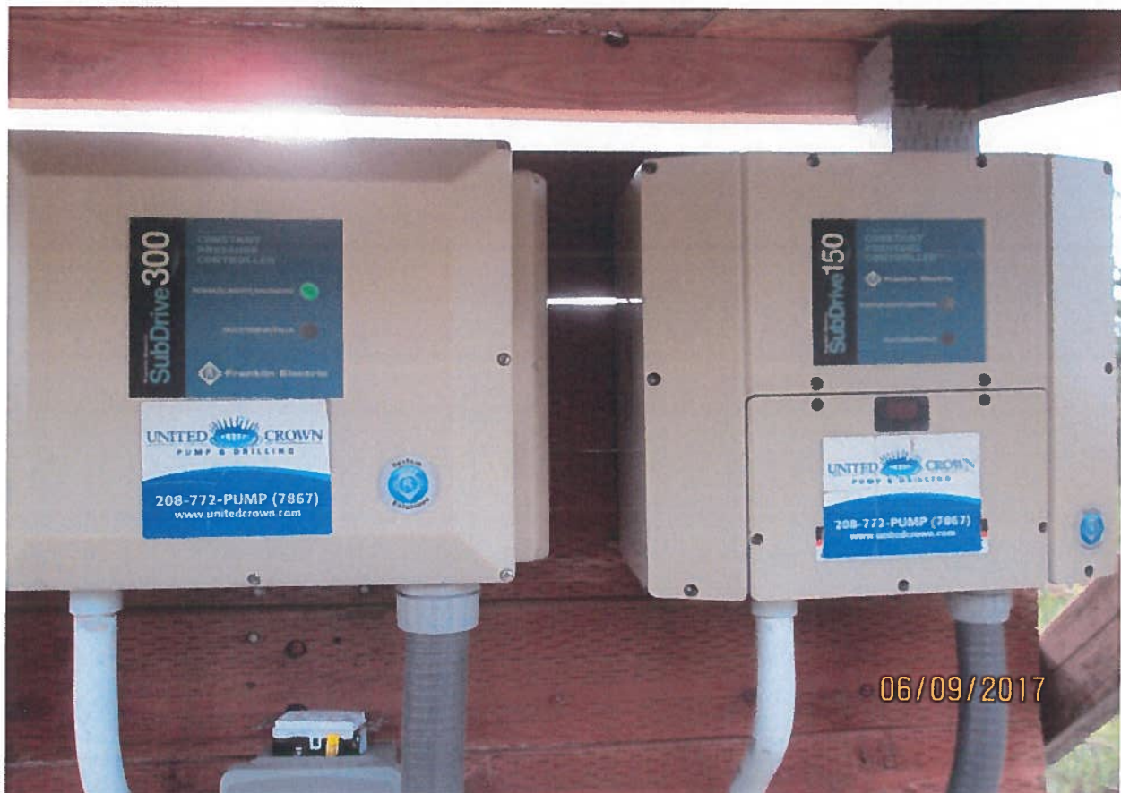
Pump control panel.
