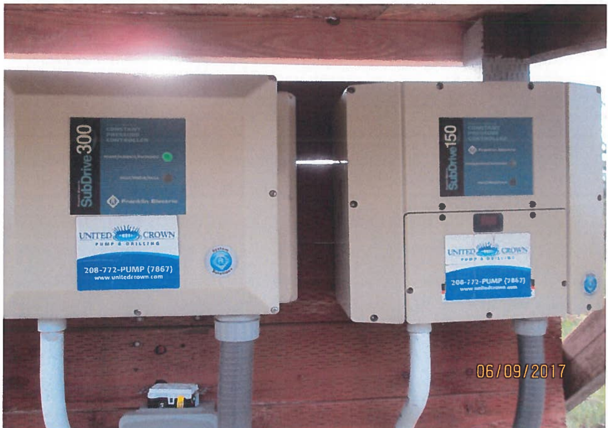
Pump control panel.
