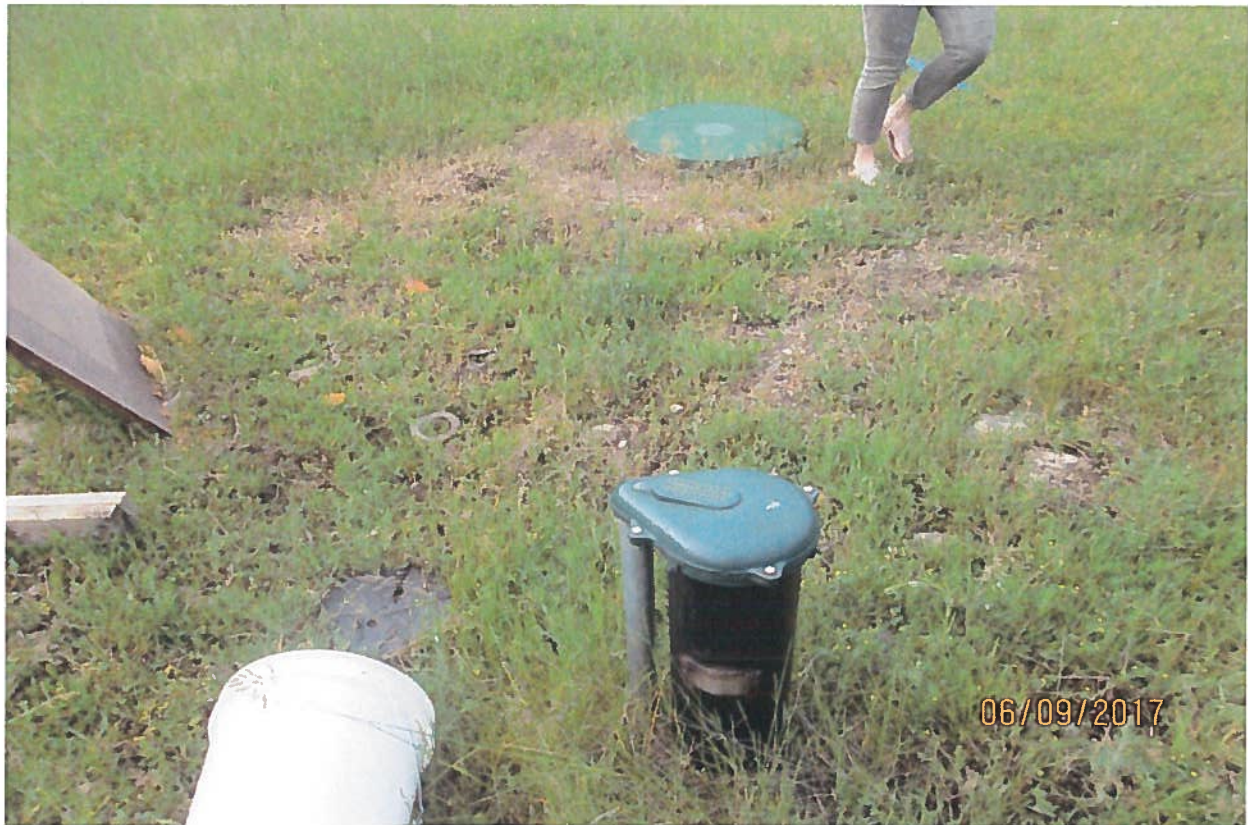
Well D0059493. 2-3k storage tank in upper portion of picture.
