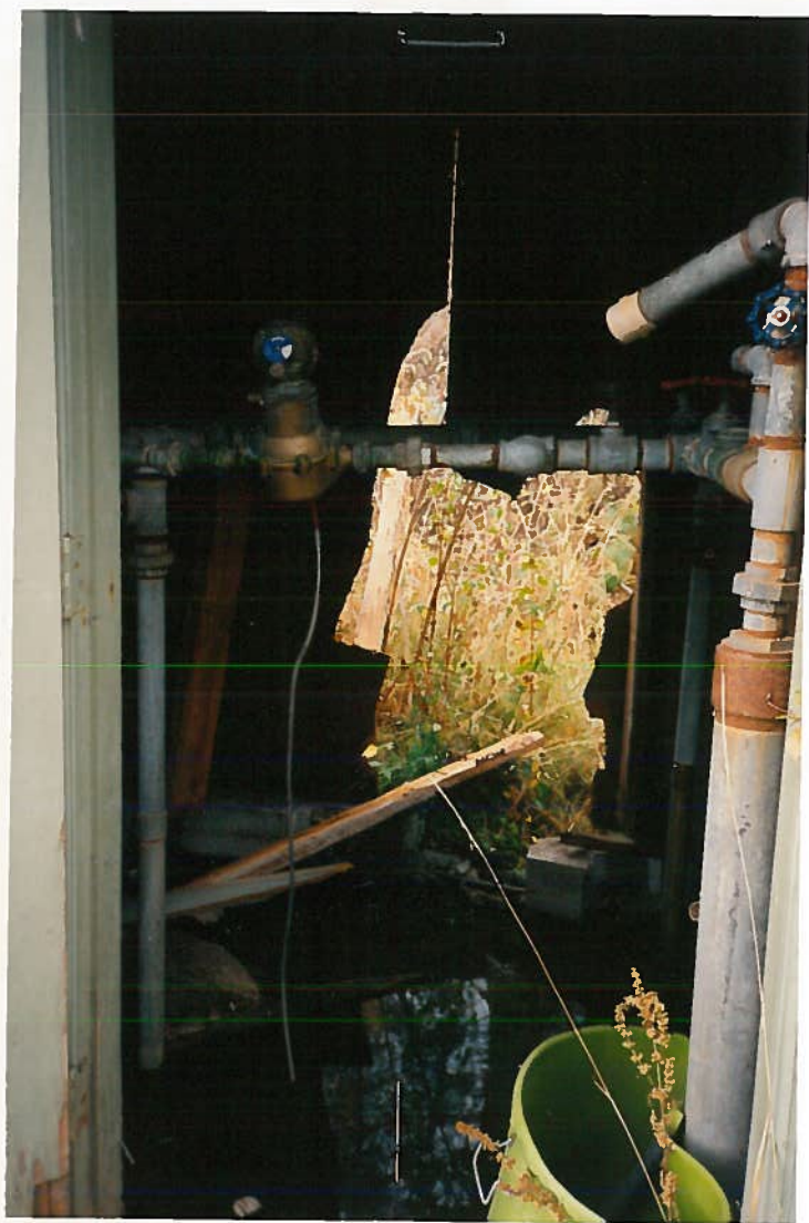
Piping from surface water POD
