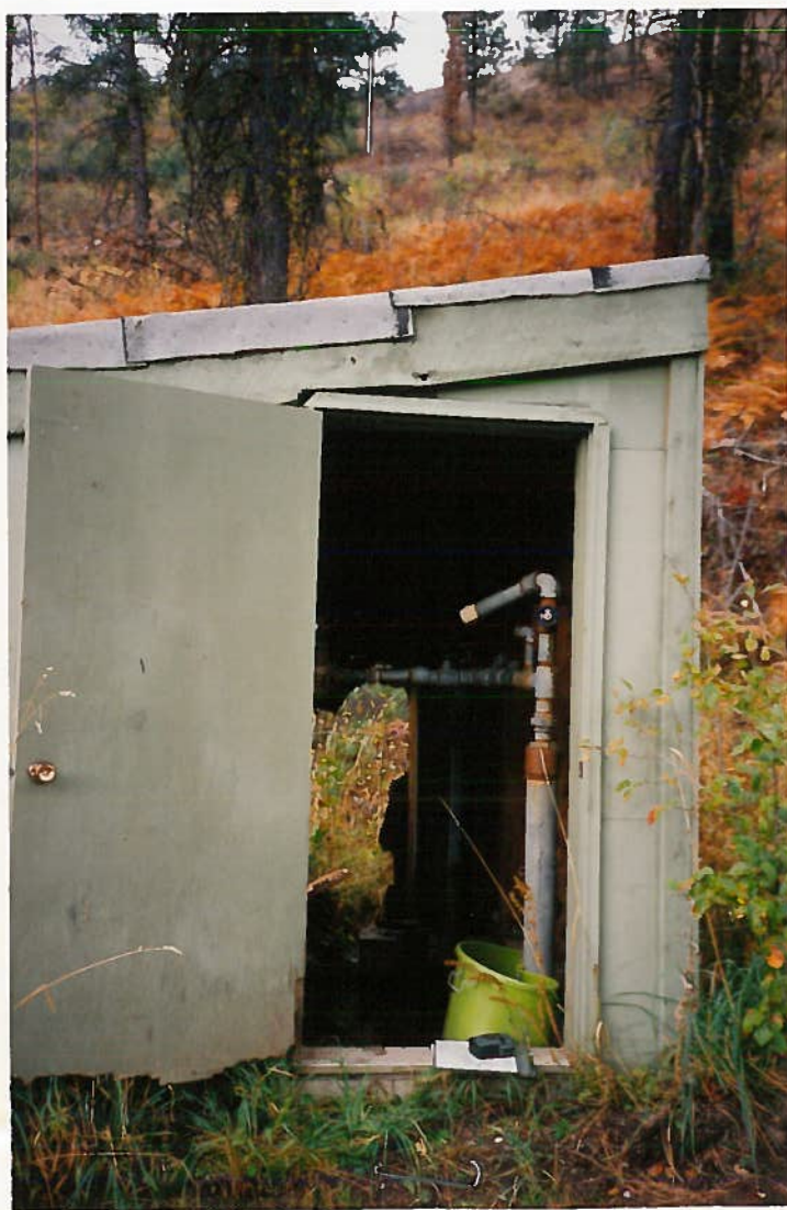
Shed where surface water and groundwater from well #1 can join and piggy-back on the same delivery system.
