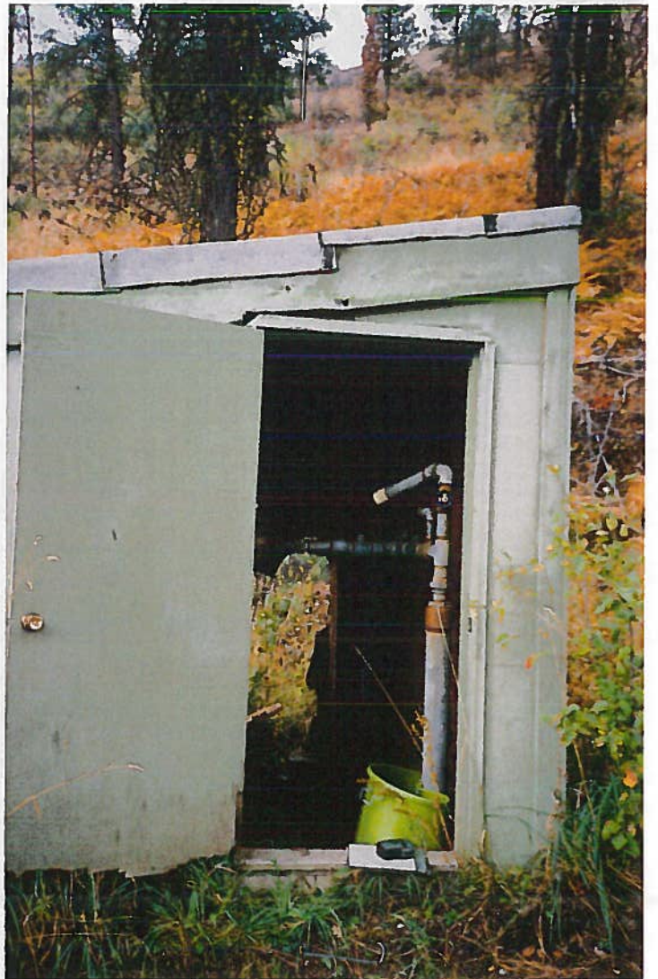
Shed where surface water and groundwater from well #1 can join and piggy-back on same delivery system.
