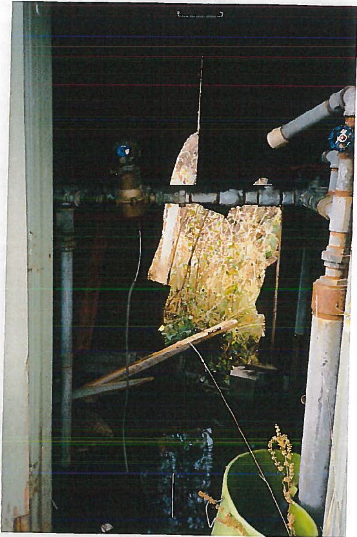
Piping from surface water POD.
