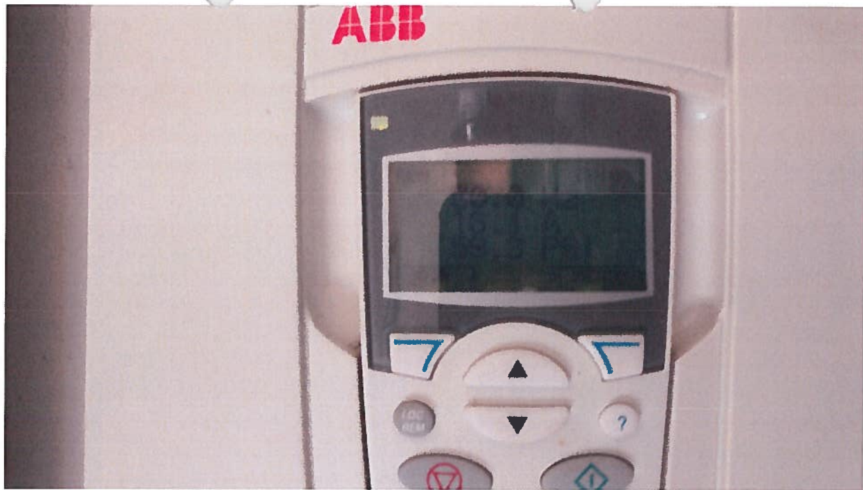
Figure 5 A closer look at the digital readout on the face of the control box.
