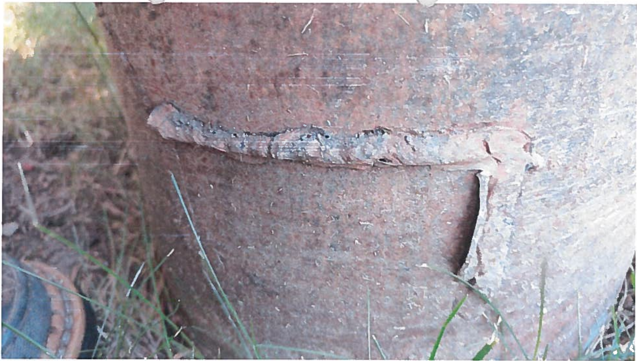
Figure 3 The weld holding the metal tag was visible, but the metal tag itself is missing from the well head.
