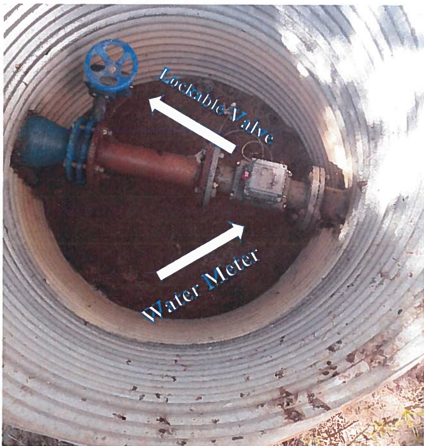
Figure 2 A view of the vault where water from the pump enters the mainline. The wheel opening the valve to the mainline can be chained in the closed position if necessary. The measuring device appears to be a propeller or turbine-type water meter.
