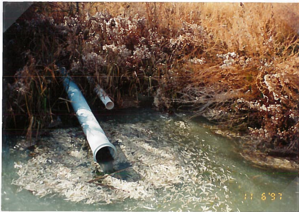
Photo showing the discharge into the first pond on the East side of the road
