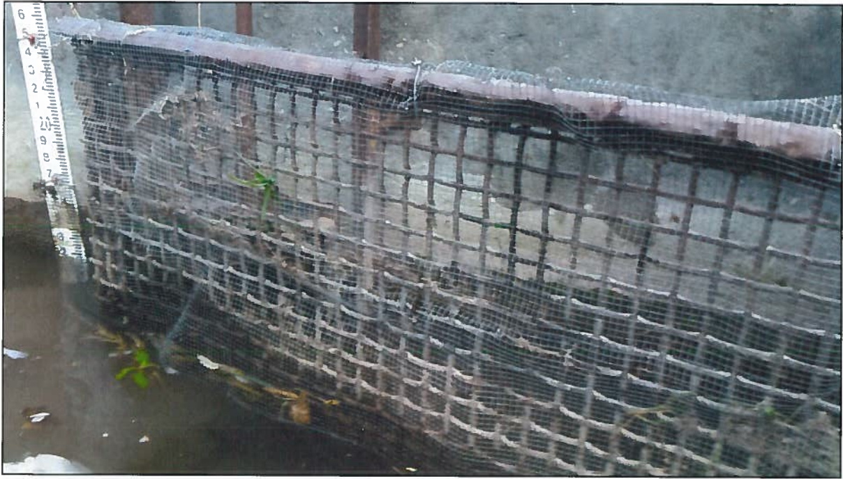
Photo A- 1. Headgate, fish screen and rated staff gage for stream measurement
