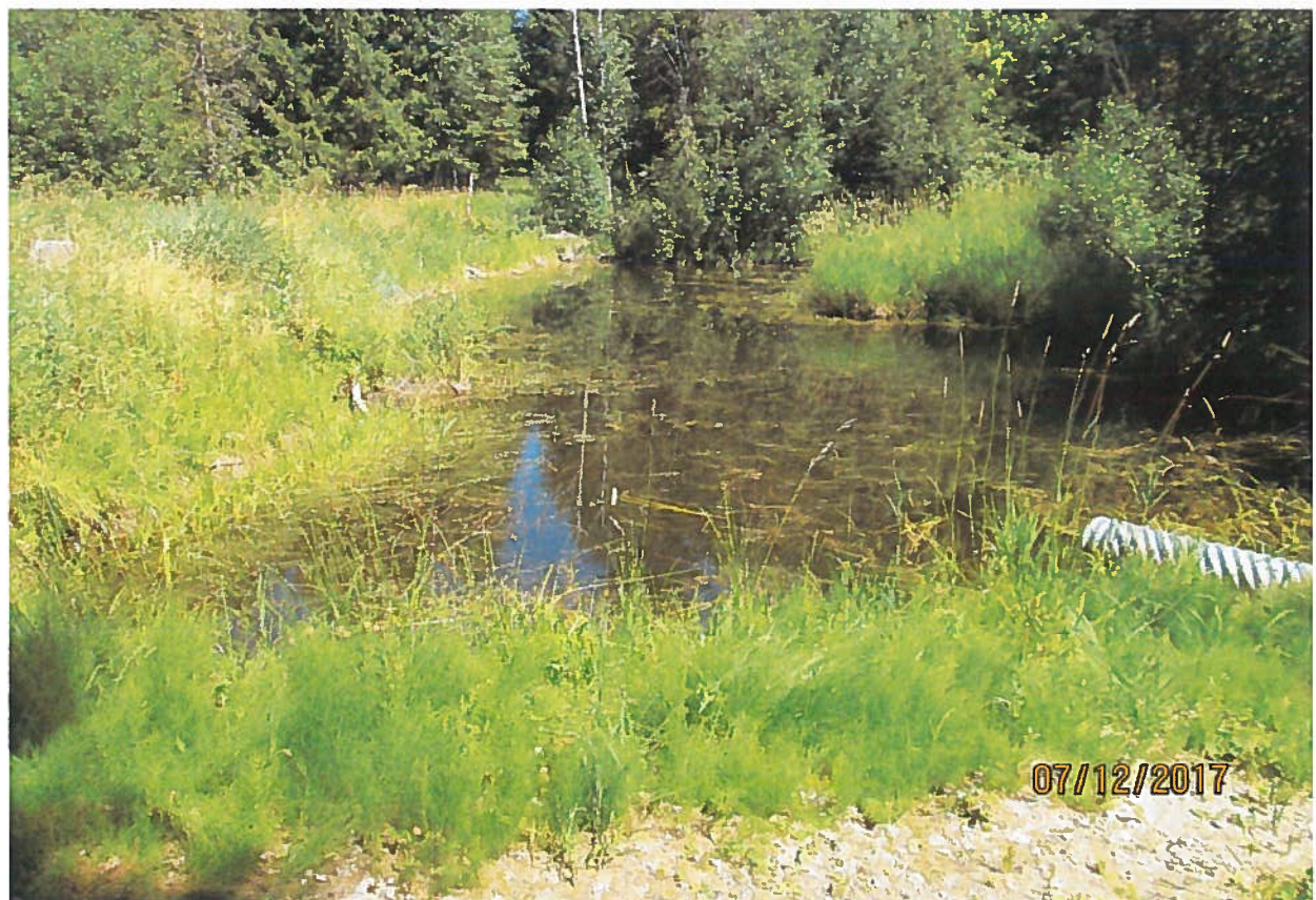
Dam to the left of the picture. Applicant had built access road across pond and put culvert underneath.
