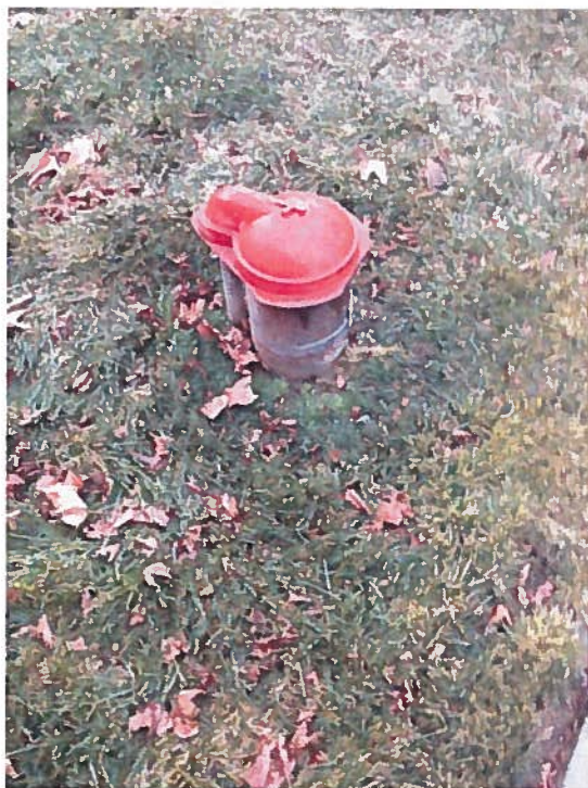
Figure 2 A second domestic well located in Gov. Lot 1 (NENE) of Sec. 3. The original intent was to run the fire protection system from this well, but it was too far from the storage tank. Now, the well is used for irrigation and fire protection without storage.
