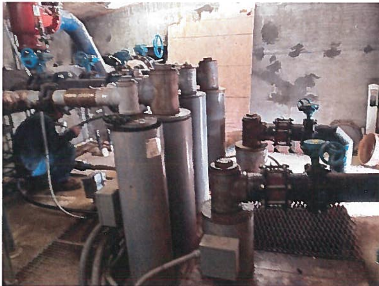
Figure 2 Inside the pump house. The well is controlled by a float valve inside a large circular vault connected to Pond 16. Four 5-hp submersible pumps divert water from the vault to the northernmost points of each of the 3 forks of the system.
