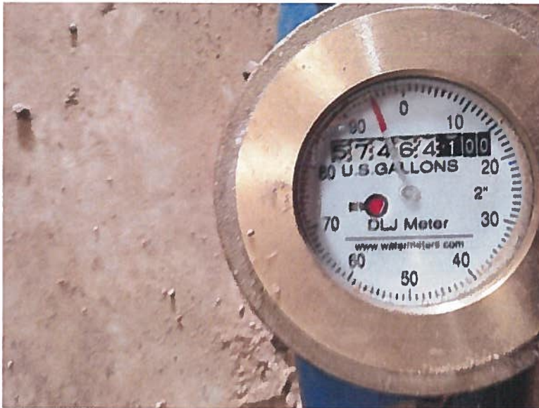
Figure 4 The flow meter located inside the pump house just up from the open discharge into the vault.
