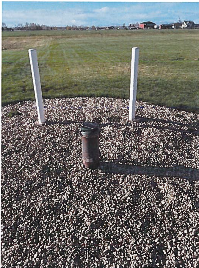
Figure 4 The domestic and irrigation well. A 1-hp pump diverts water to 20 sprinkler zones and to the church building for restrooms and sinks.
