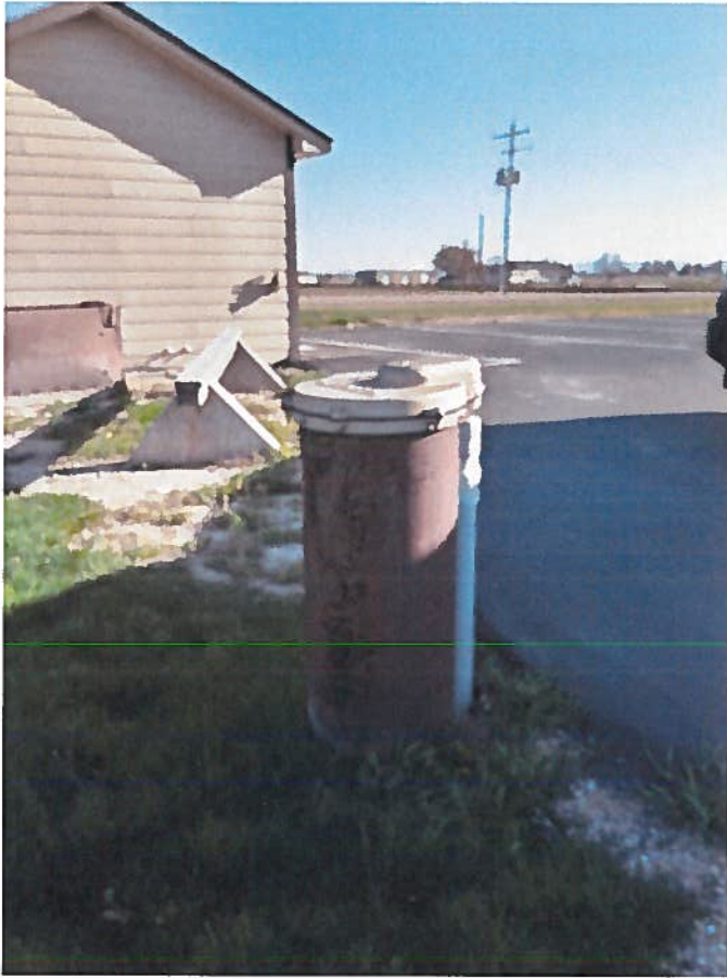
Figure 1 This fire protection well has a 75-hp pump with a 17-hp booster. It supplies water to both a fire hydrant, and to the internal sprinkler system for the church.
