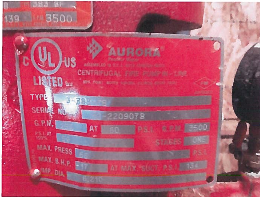
Figure 3 The information for the booster pump.
