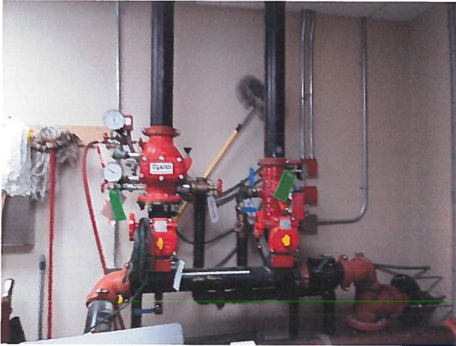
Figure 7 The internal sprinkler system controls.
