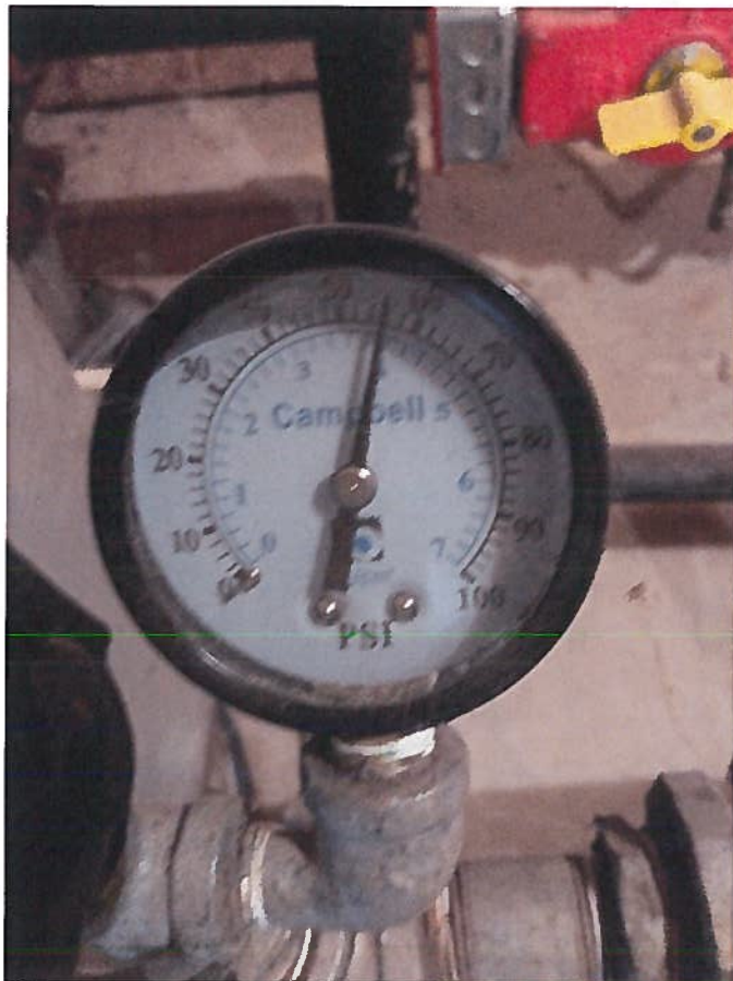
Figure 5 A pressure gauge showing a system pressure of 55 psi for the irrigation and domestic system.
