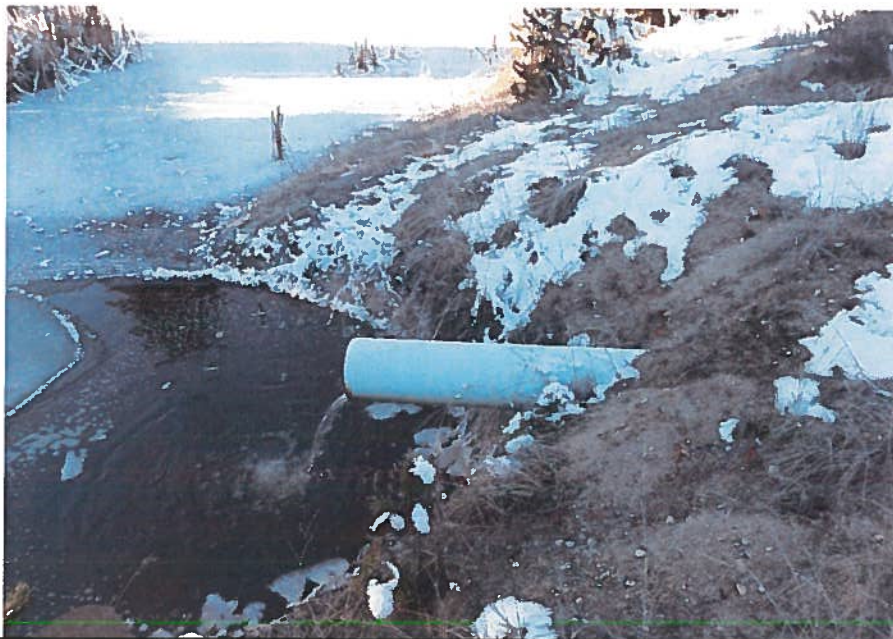
Figure 5 A PVC outlet running into the second pond at WPT 180. The pipe is supposedly hooked up to the recirculation pump to the south. The pump was not running at the time of the exam, but water was coming from this pipe. According to the owner, the source of the water is runoff from the surrounding landscape.
