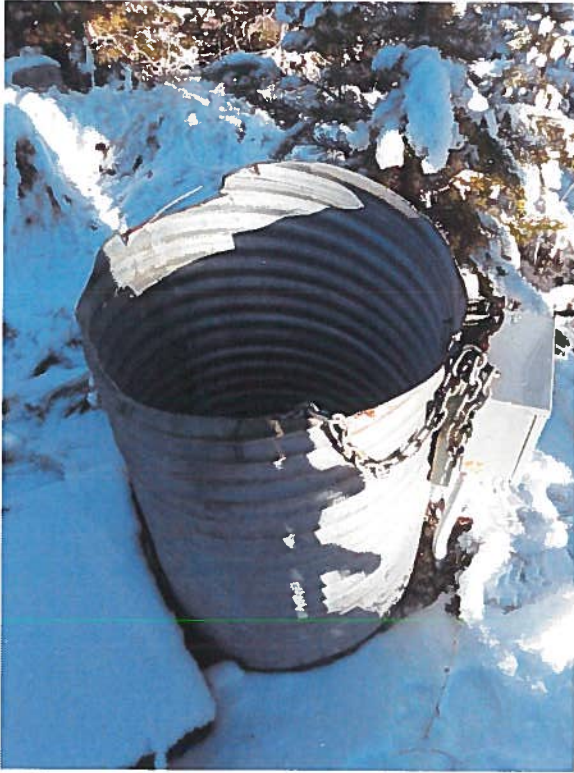
Figure 1 The vault with recirculation pump located at the southernmost pond at WPT 177 on the system diagram.
