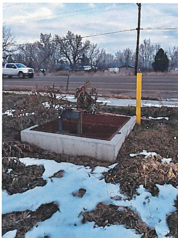
Figure 5 The pump house where irrigation water is taken from the northwestern pond and distributed throughout the subdivision. Irrigation and evaporation water is provided through surface water shares from the New Union Ditch Co.
