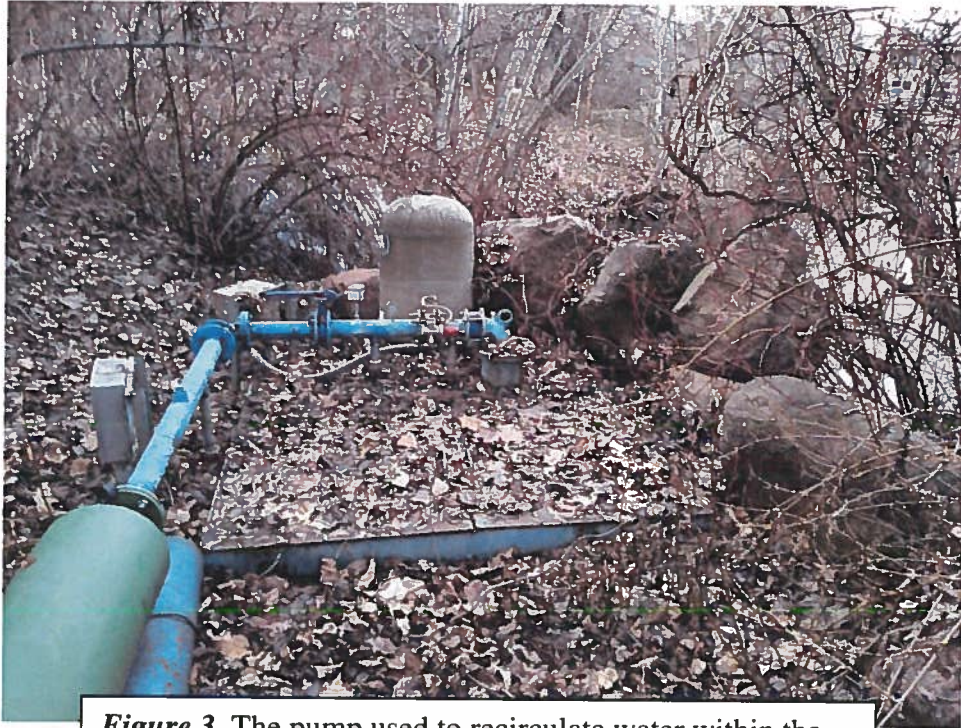
Figure 3 The pump used to recirculate water within the system.
