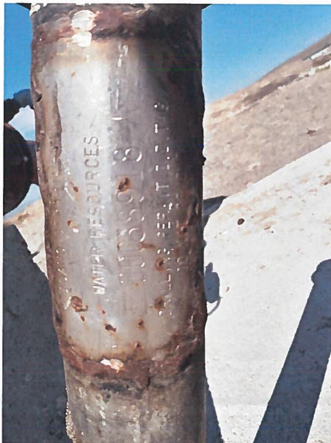
Figure 1 The point of diversion is a 12 3/4" well with a 50-hp Layne-Bowling pump.
