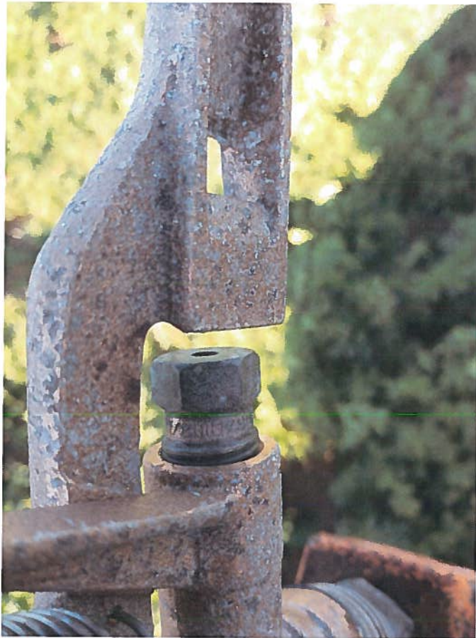
Figure 5 A total of 85 sprinkler heads w/ 1/8" nozzles are distributed throughout the 3 wheel lines.
