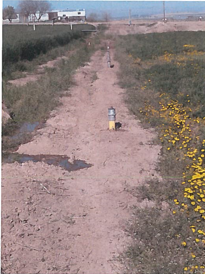
Figure 3 3" risers from the mainline to hook up to wheel lines.
