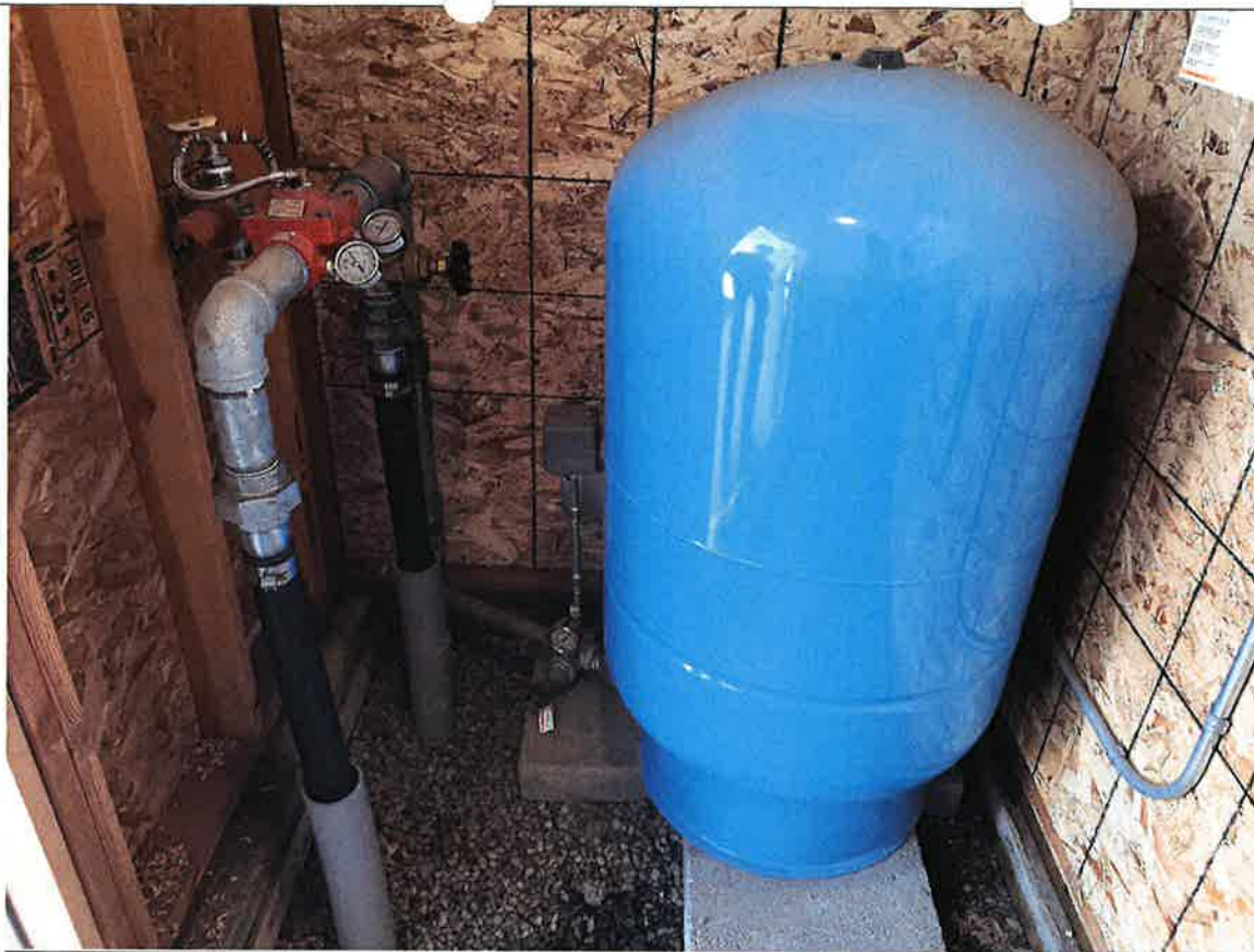
Pressure tank and delivery system that is ran at no more than 55 psi.
