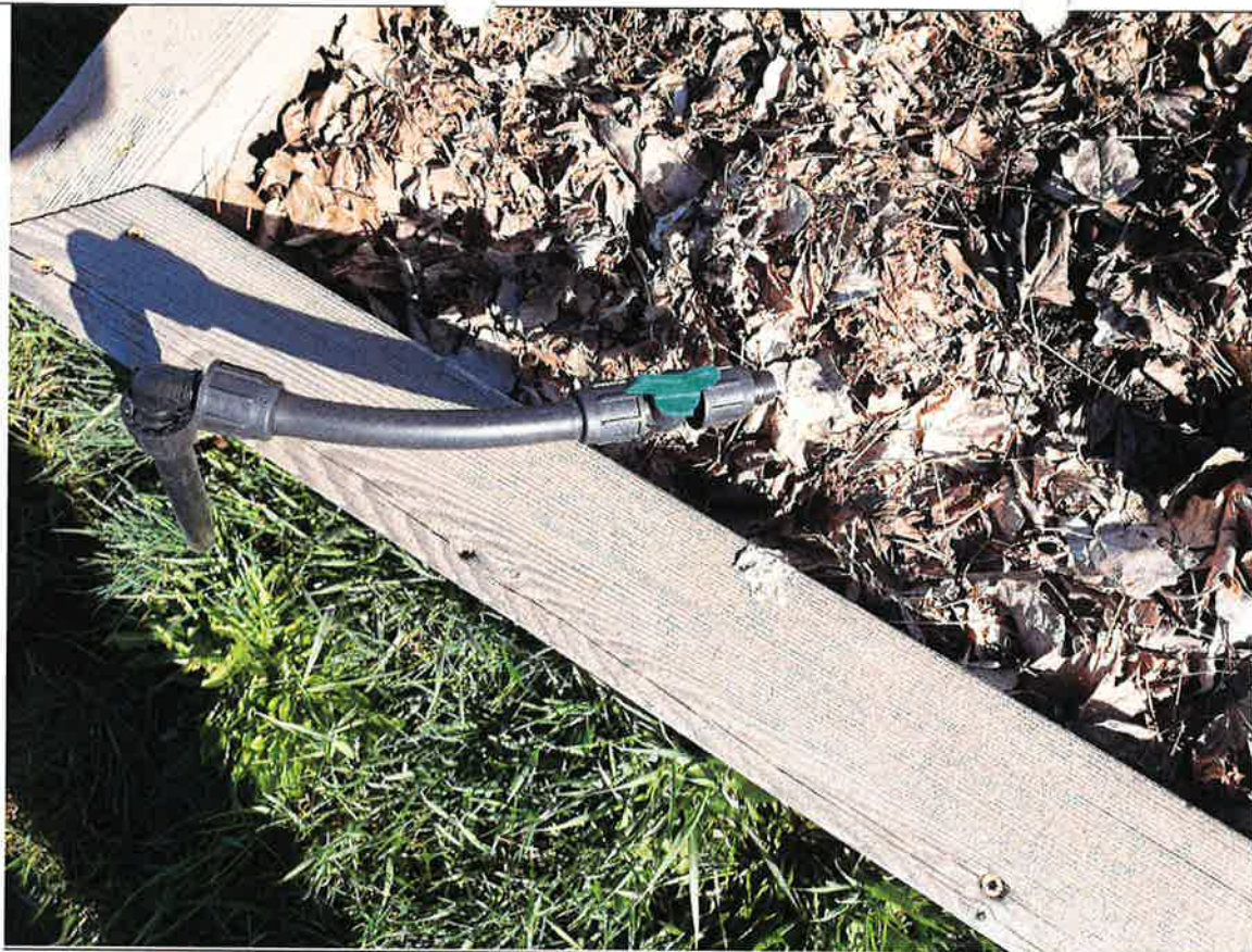
Up close view of the hand valve attached to the funny pipe.
