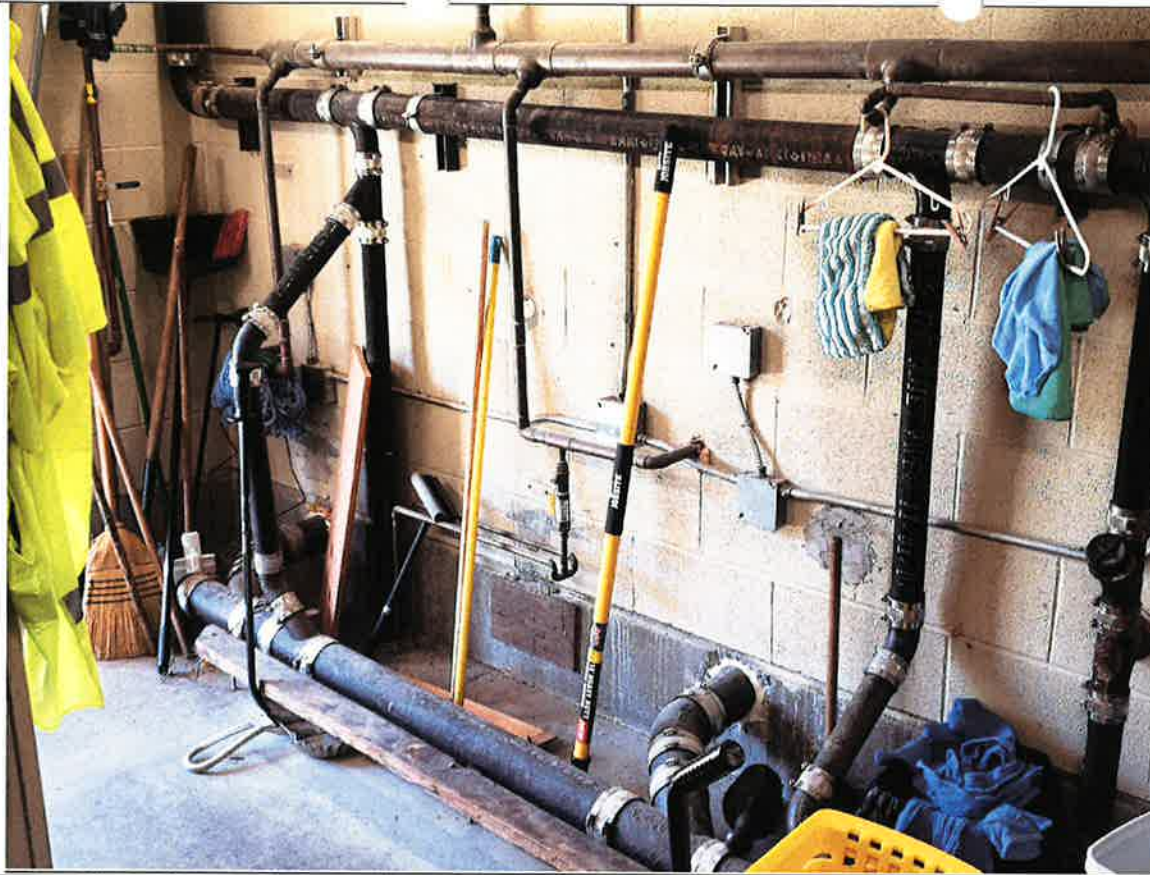
Water and sewer lines to all the fixtures.
