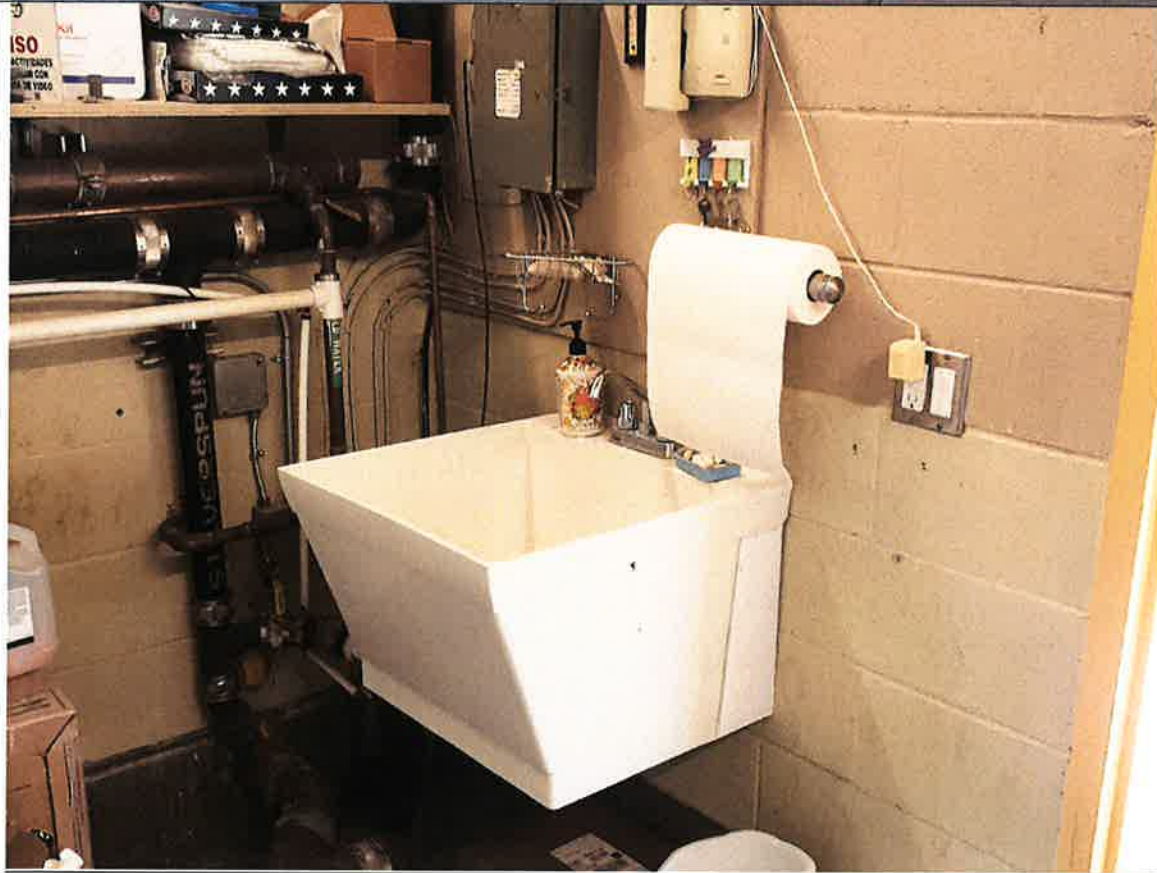
Maintenance sink in the pump room behind the restrooms.
