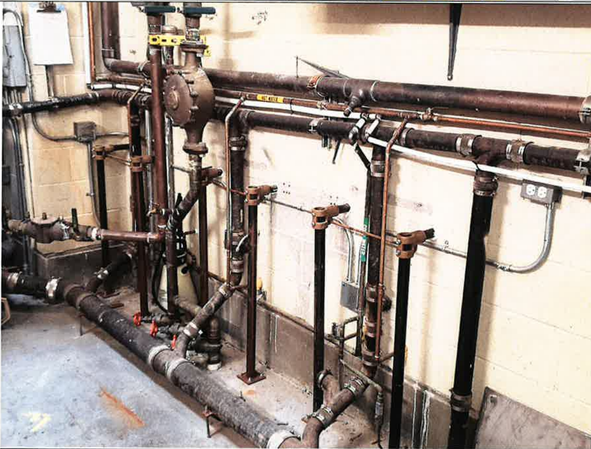
Water and sewer lines to the fixture in the women's bathroom and irrigation totalizer.
