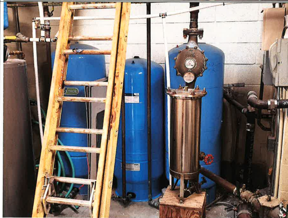
Three pressure tanks and domestic totalizer.
