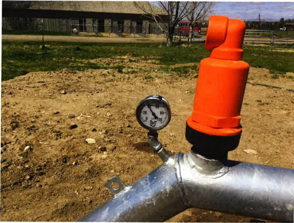
Pivot delivery pipe pressure
