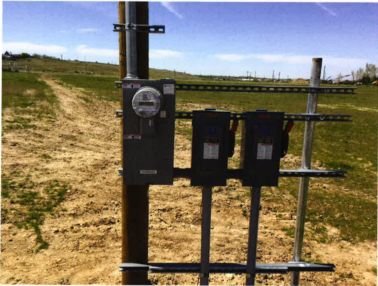
Meter base and disconnect switches (follow up photo taken by examiner on April 25, 2018)
