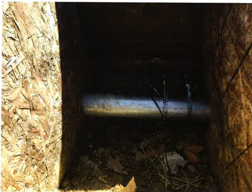
Portable flow meter installed on 4-inch discharge pipe from well
