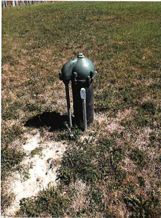
Figure 1 An 8" well drilled in 2014 to replace one of the original wells which is no longer in use. This well has a 15-hp pump which diverts water through a 4" line to 2 1000-gallon tanks.
