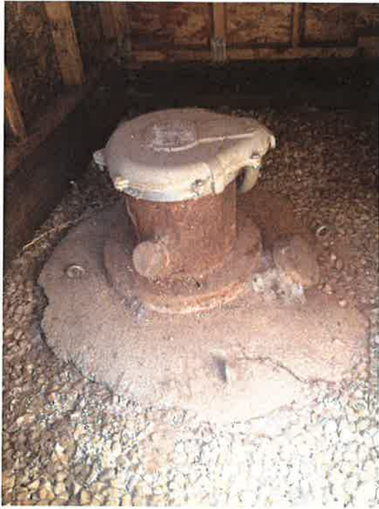
Figure 3 The 16" well with a 20-hp pump. There is no record of this well in the IDWR database. TDH for this well was assumed to be the same as the well in Figure 1 for system capacity calculations.
