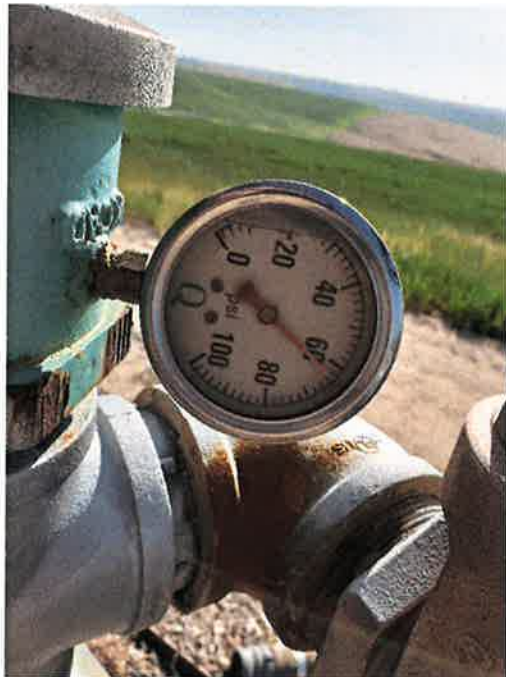
Figure 5 60 psi in the main 8" line to the pivot center.
