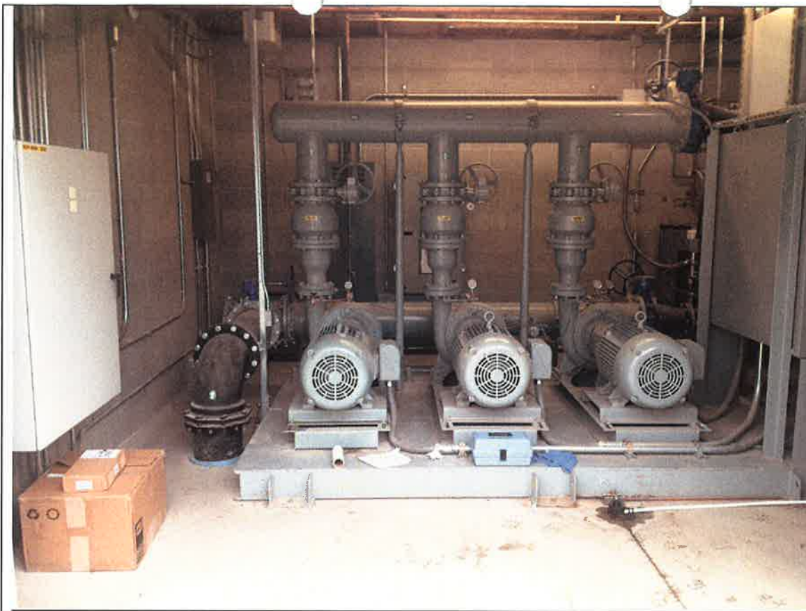
Pump house with three booster pumps.
