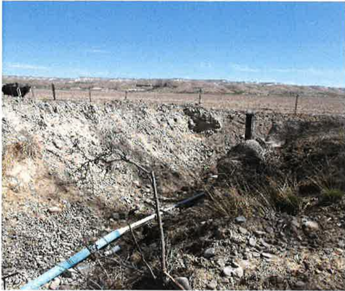
Collection pipe and casing for pump
