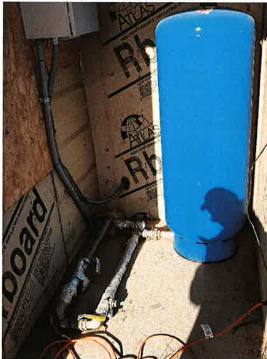
Figure 2 81-gallon WellMate pressure tank located in the pump house with the irrigation timer.
