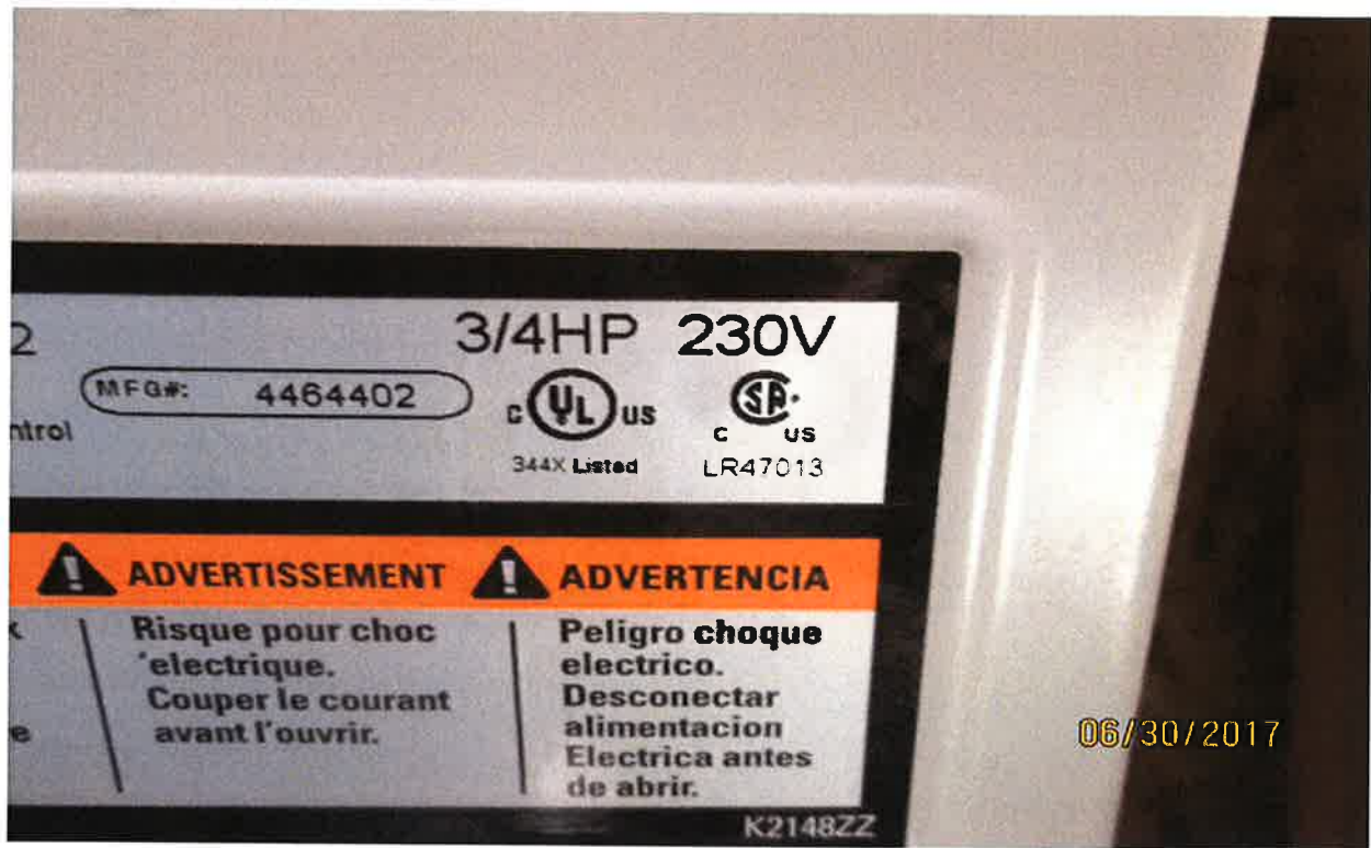
¾ hp pump in well. Unable to perform flow measurement because it was pumped directly to pressure tank.
