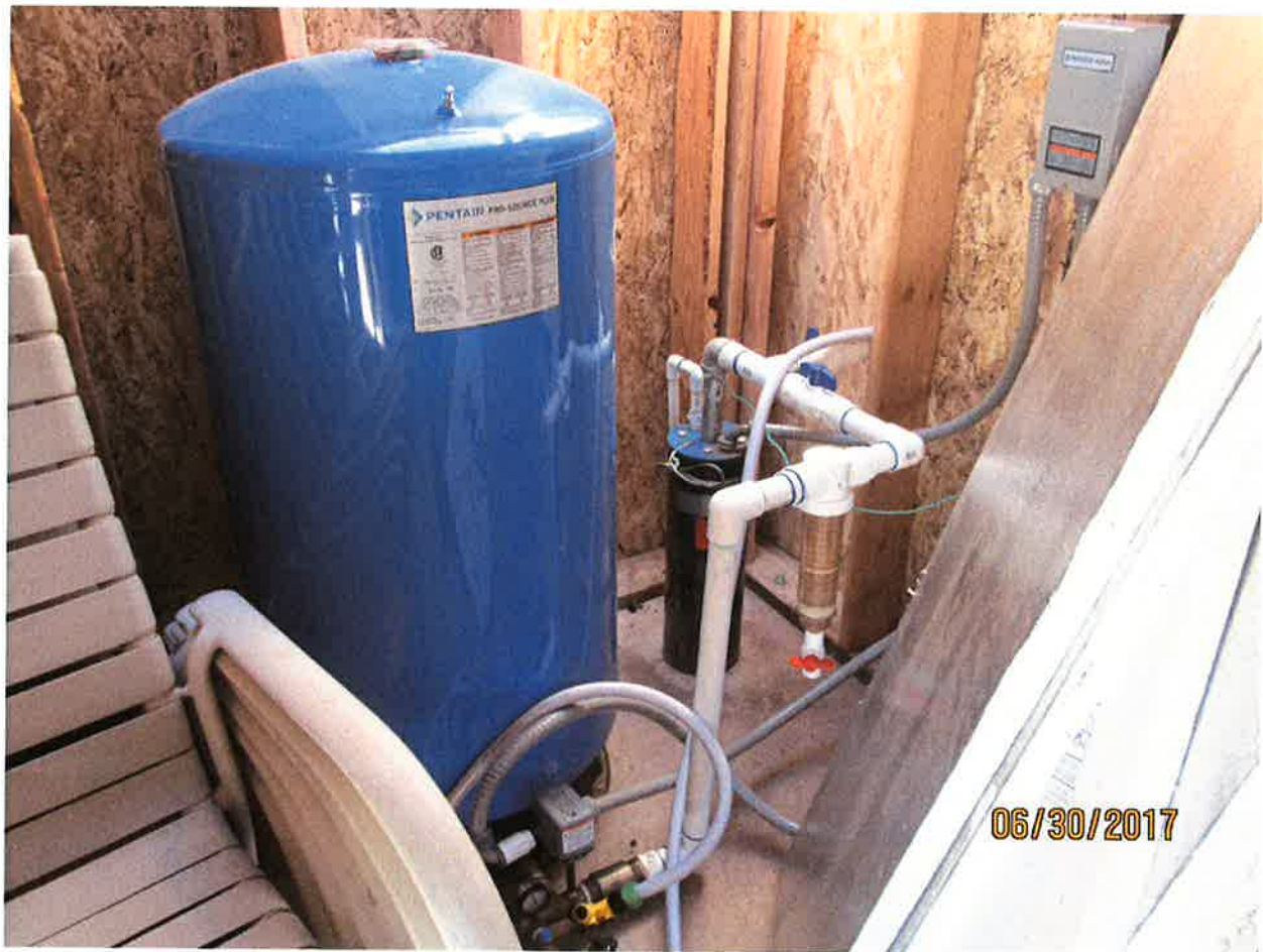
Inside pump house with piping to pressure tank.
