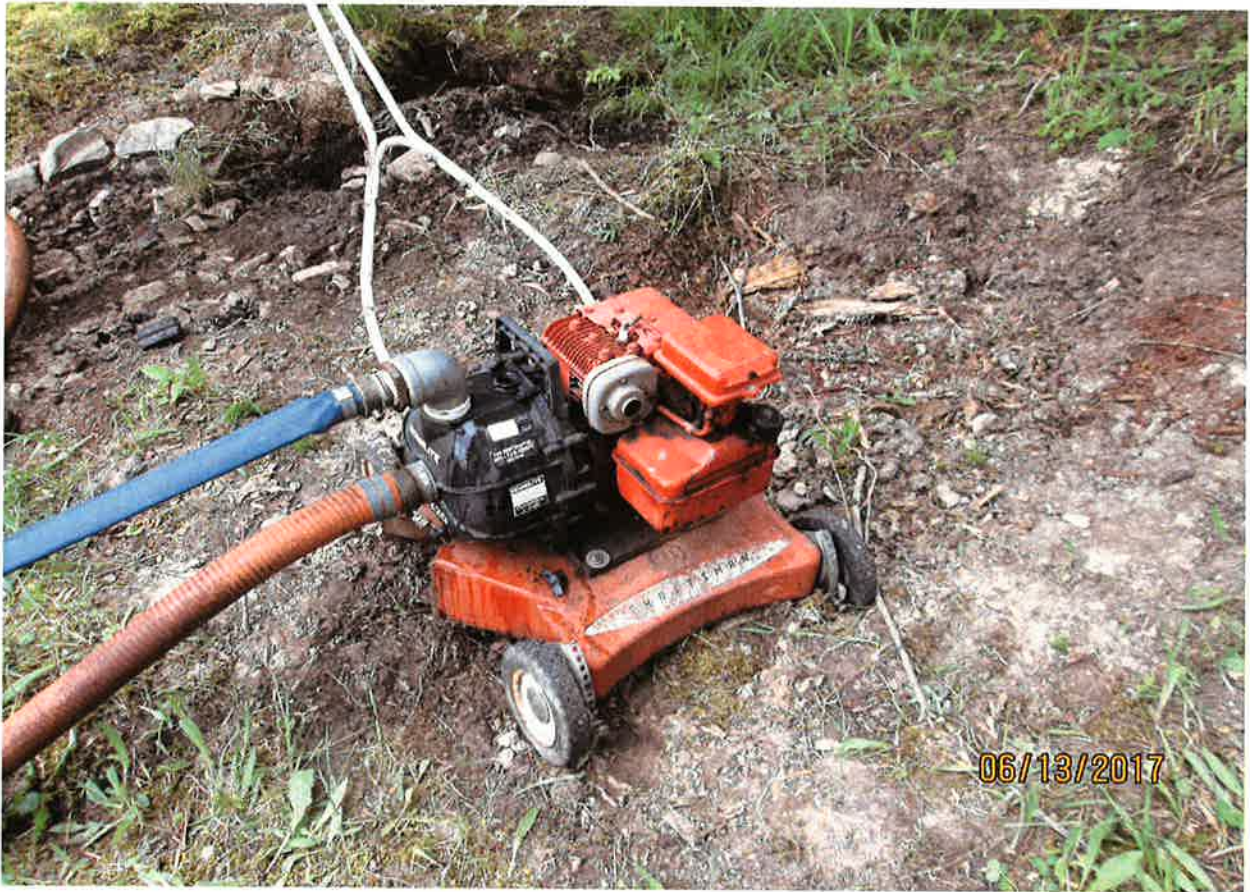
Portable pump applicant had built for irrigation.
