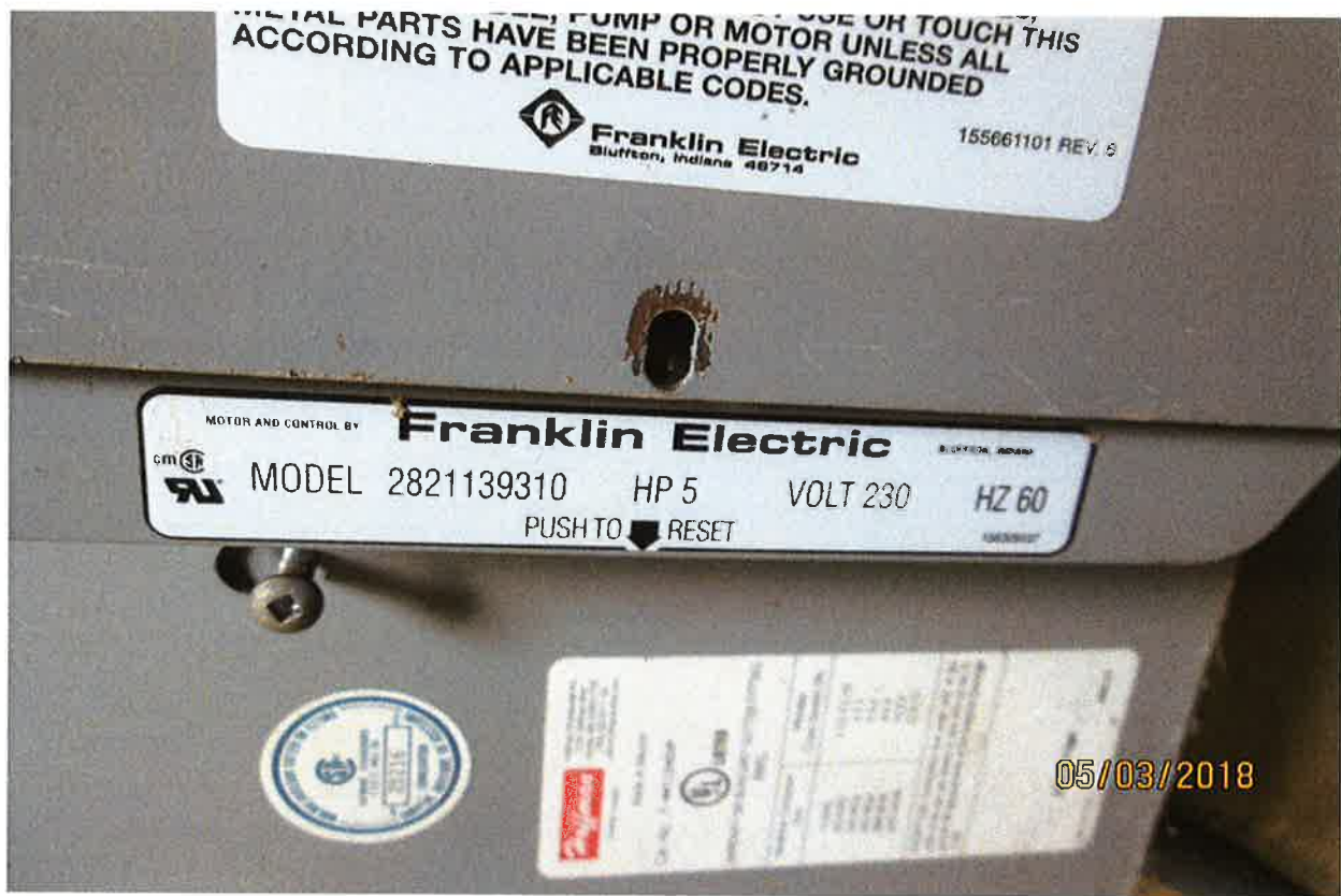
5hp pump in well.
