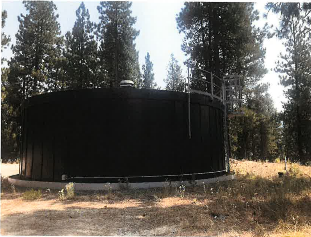
Domestic Storage tank
