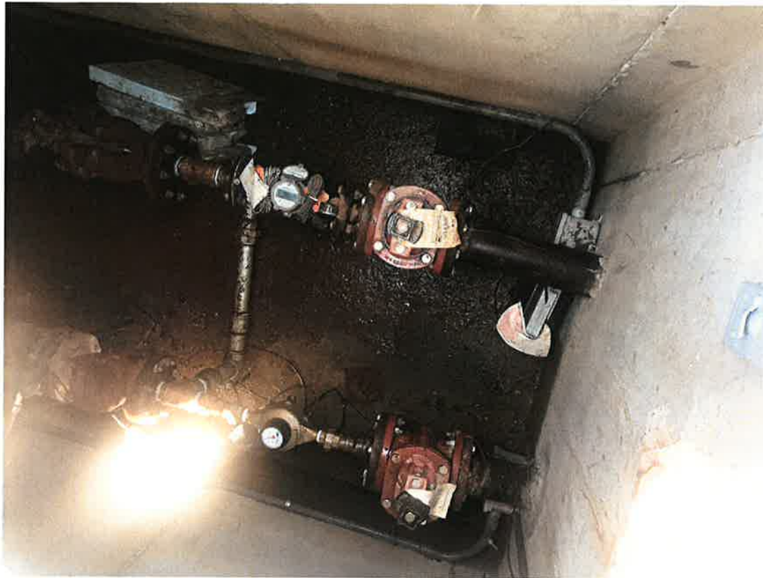
Looking down on pump vault with in-line flowmeters.
