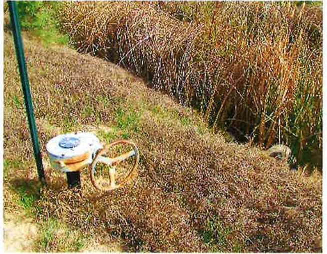
Typical slide gate used to divert water into ponds 1, 2 and 3 from the ditch on the eastern side of the ponds
