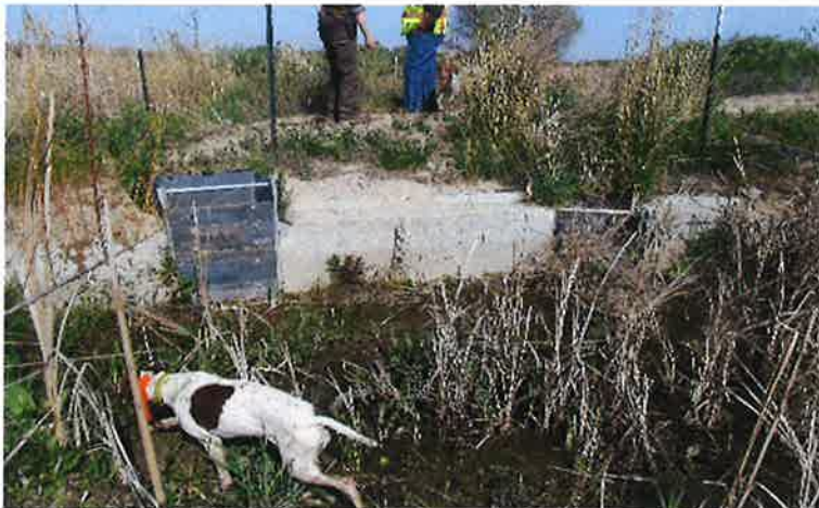
Slide gate used to allow flow between ponds
