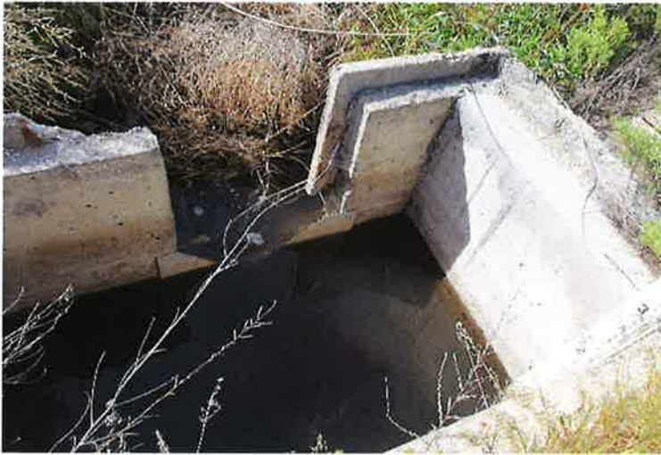
V-notch weir at permit holder's diversion from Bruneau Buckaroo Ditch
