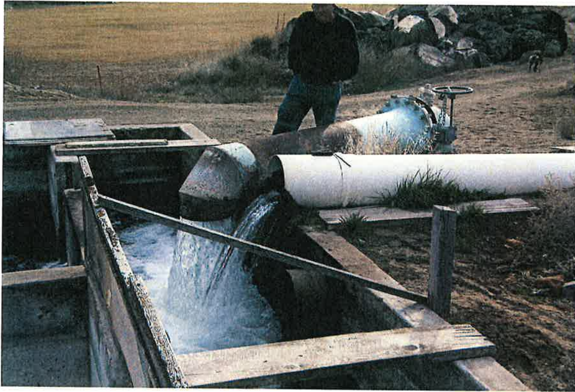
Photo taken when water was being diverted from three different sources. White plastic pipeline comes from Porcupine Springs. Metal pipeline comes from Alpheus Creek Springs. Lower concrete pipeline comes from Perrine Coulee.
