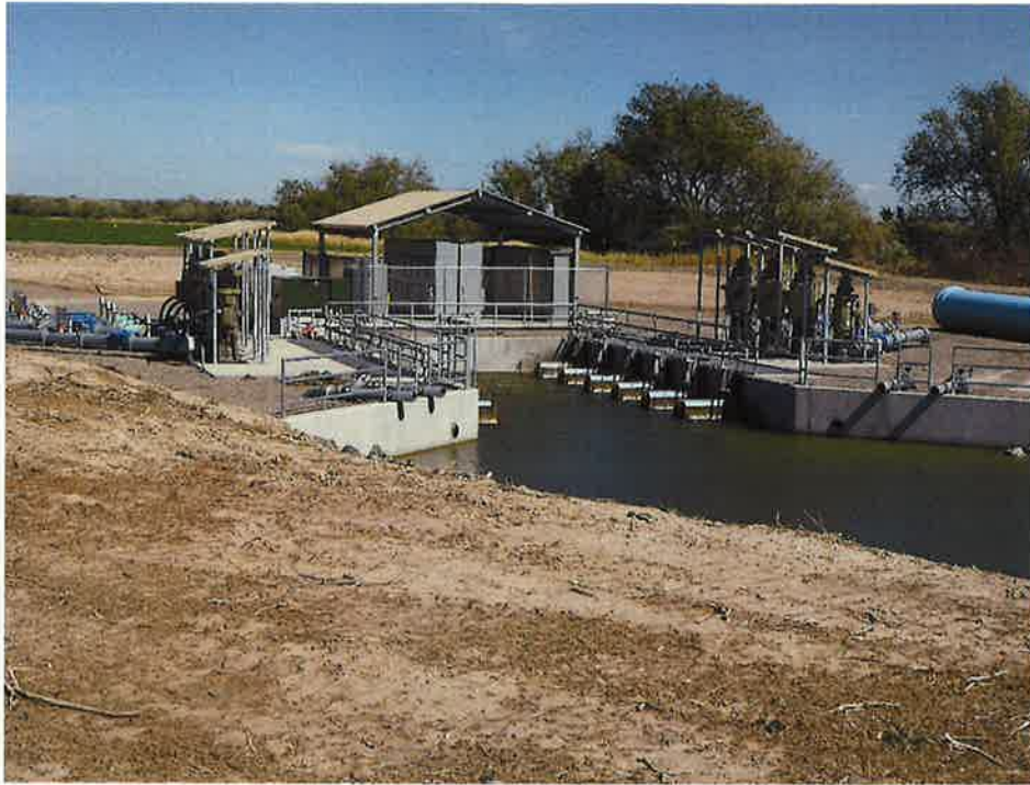
A&B Pumping Plant #2
