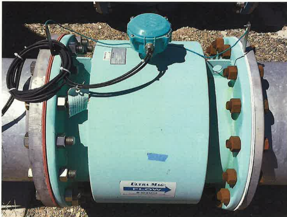
Typical Meter Installation
