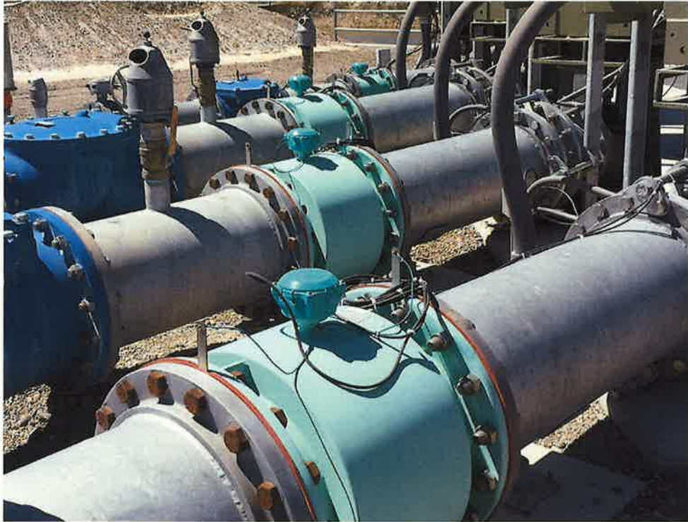
Meter Installations on One Bank of Pumps
