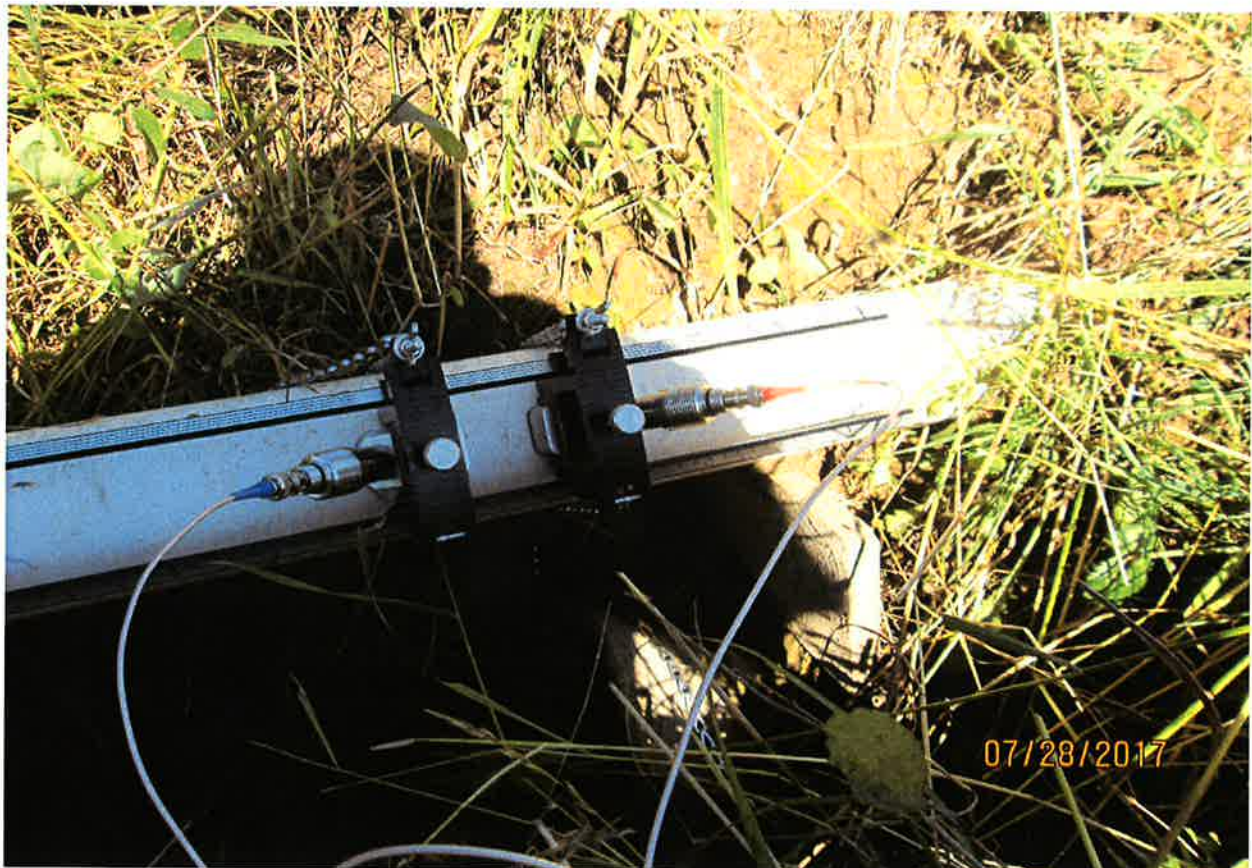
Flow measurement performed using GE Panametric Meter.
