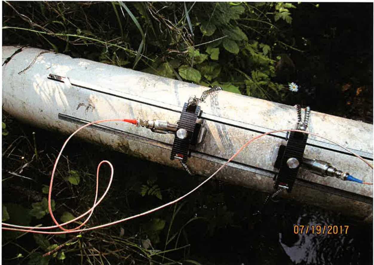
Panametric Flow Meter used to conduct measurement.
