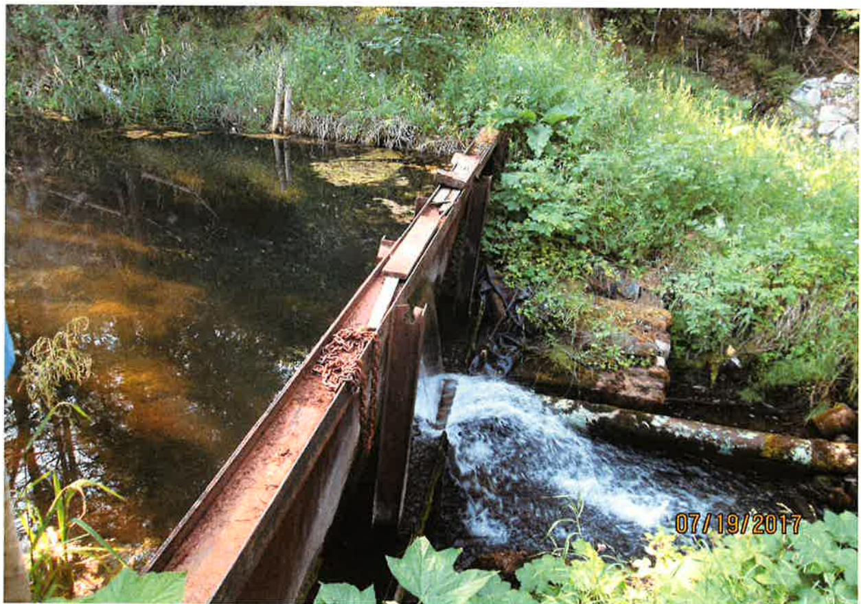
POD on Sand Creek. Applicant had built 5 foot dam.
