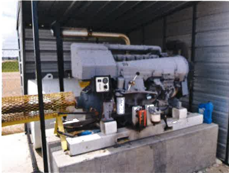
Figure 3 Diesel engine used to drive the turbine pump.
