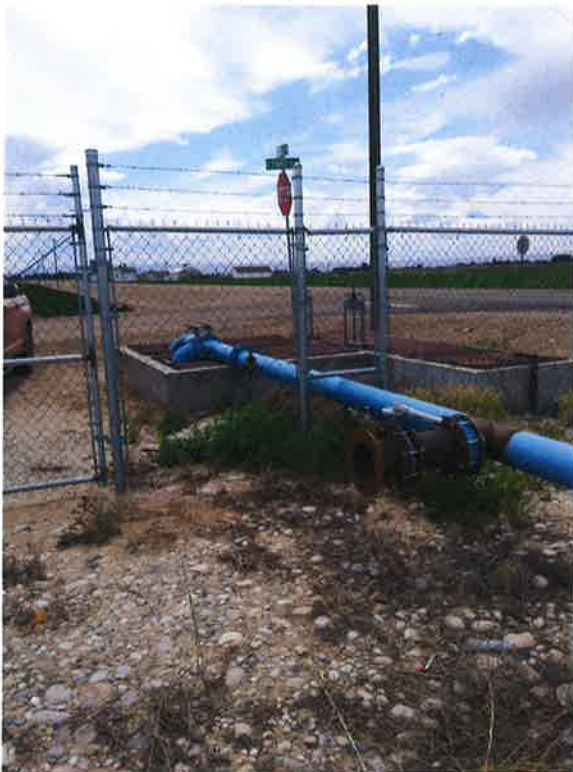
Figure 4 8" line open discharge to open ditches to irrigate under this right and 63-33759
