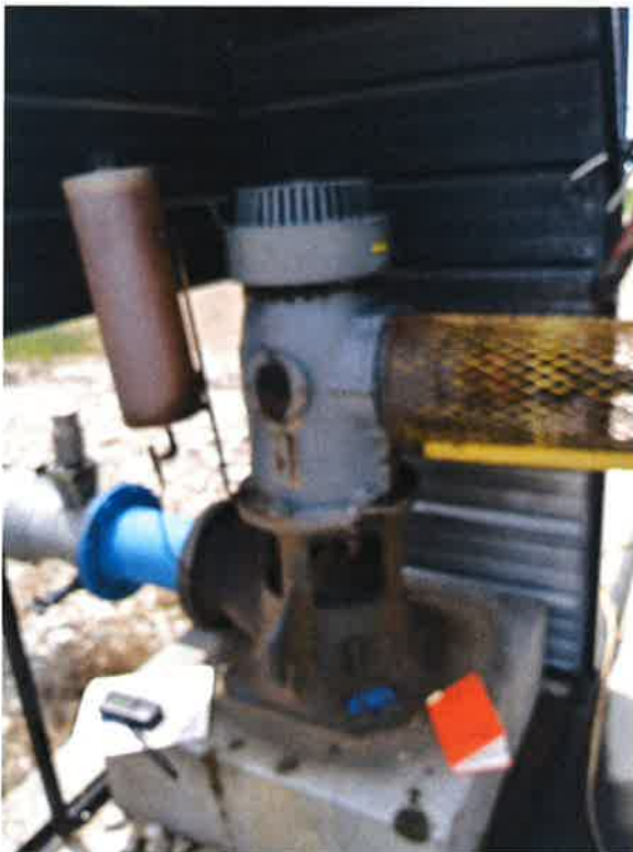
Figure 2 Turbine pump driven by diesel engine used to divert water from the well. 8" discharge line.
