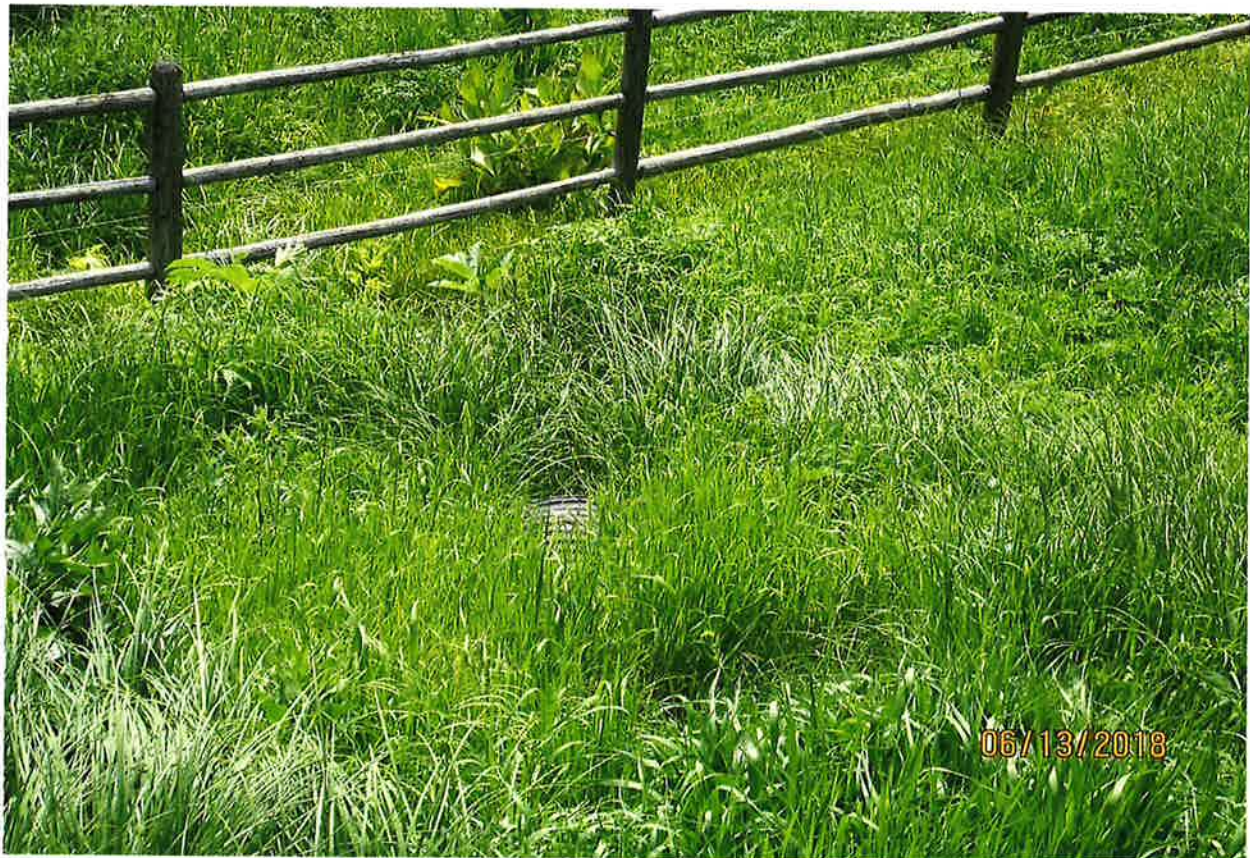
Outflow culvert to unnamed stream and then Buffalo Gulch Creek.
