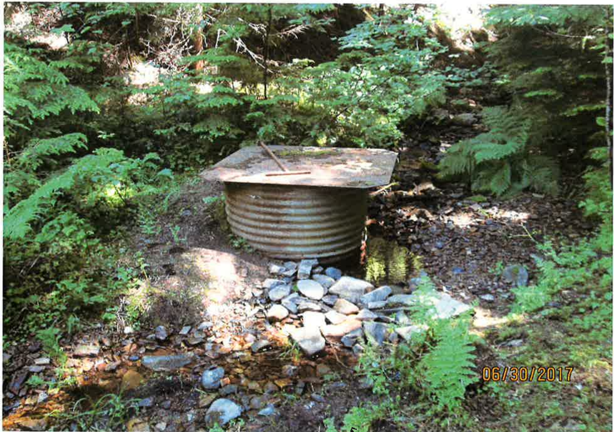
Applicant had put in culvert adjacent to stream for diversion system.
