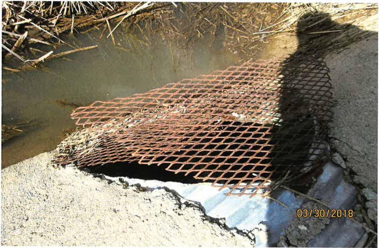
Outflow culvert screened to prevent clogging and fish escaping.
