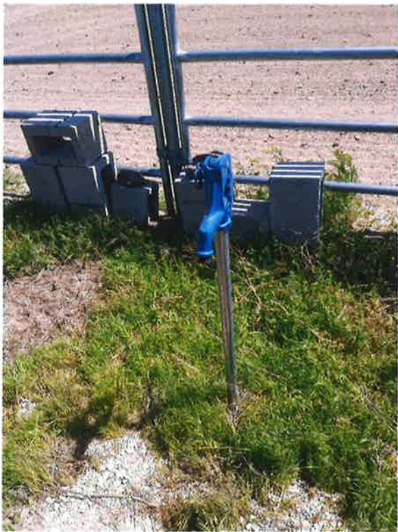
Figure 4 One of five hydrants used to fill stock tanks and water the garden.
