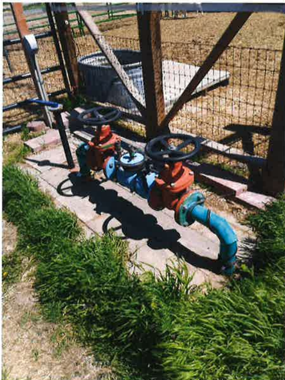
Figure 6 Backflow preventer and control valves on the irrigation supply line.
