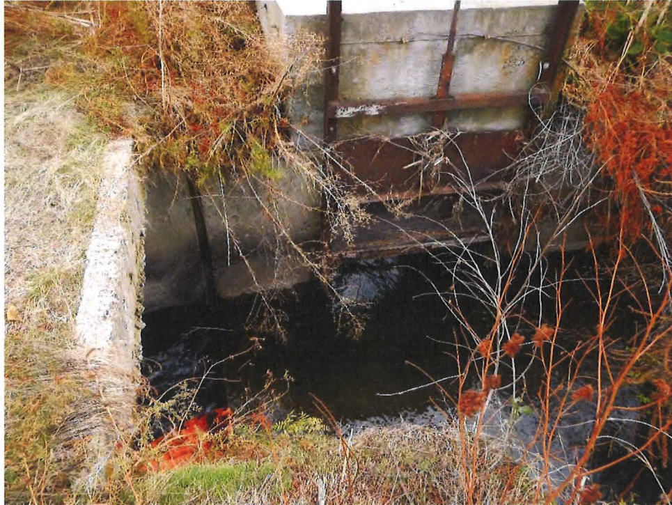
Photo 4. Gate to control the amount of water entering the Wilson ditch in center and overflow structure to control water returning to Little Willow Creek on left
