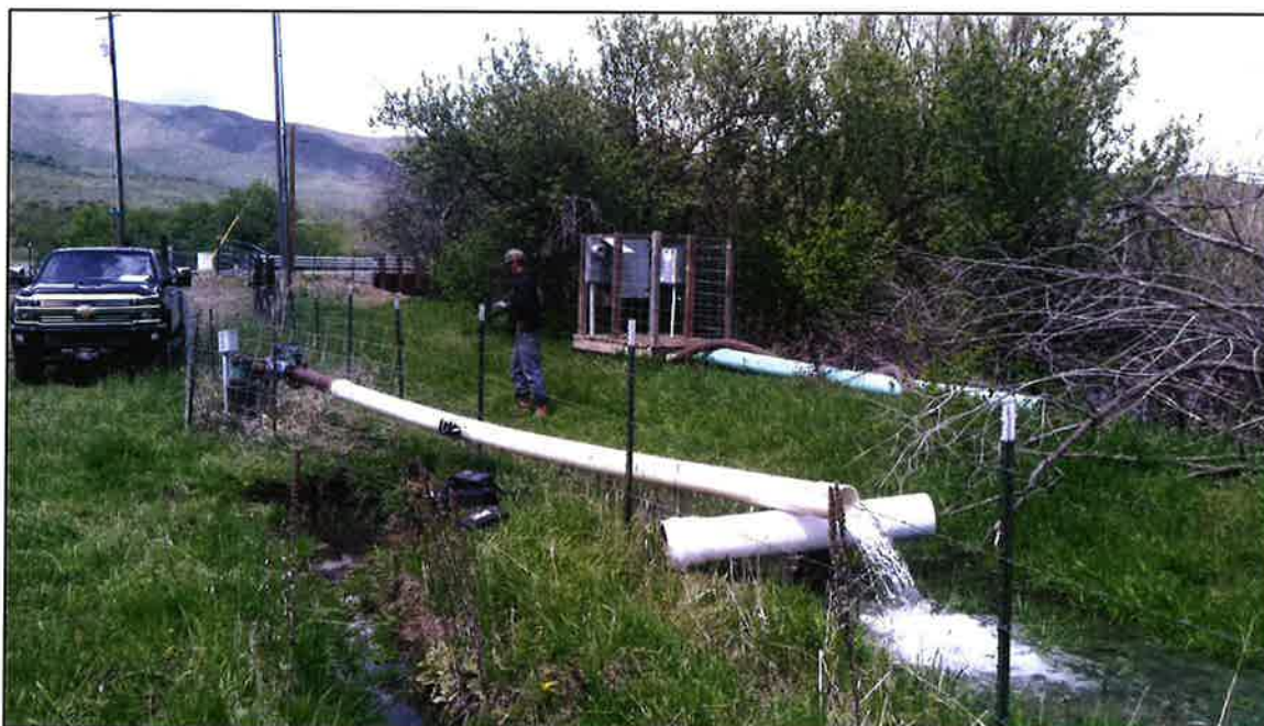
Figure 4: Well being pumped with flowmeter mounted on 6-inch PVC pipe about 12 feet downstream of the well head. PVC pipe was temporary for the flow measurement and water is normally directed to the ditch on left.
