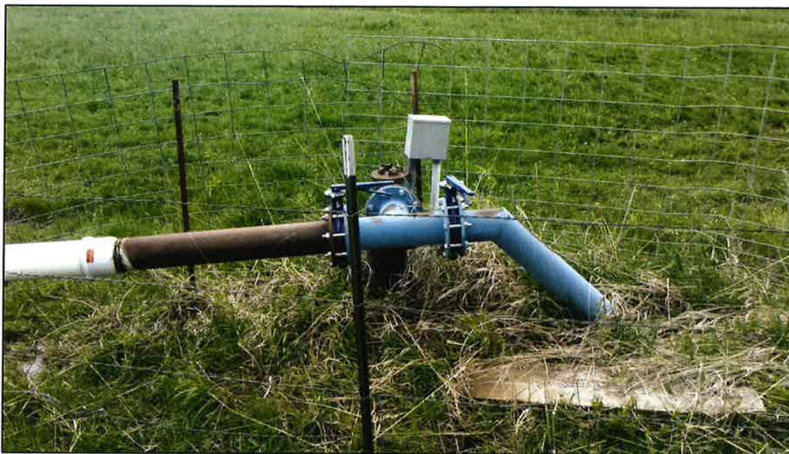
Figure 3: Well and discharge piping. The pipe on left discharges to the ditch along the field's northeast side. The pipe on right discharges to the ditch along the field's west side. All flow diverted to the left pipe during exam.
