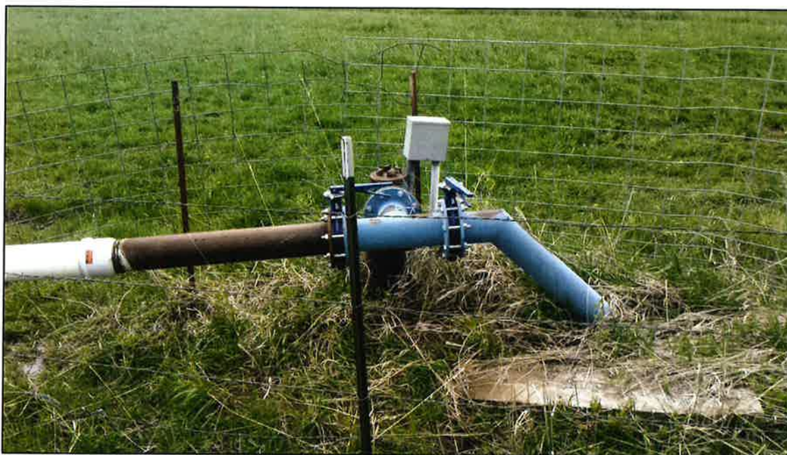
Figure 1: Well and discharge piping. The pipe on left discharges to the ditch along the field's northeast side. The pipe on right discharges to the ditch along the field's west side. All flow diverted to the left pipe during exam.
