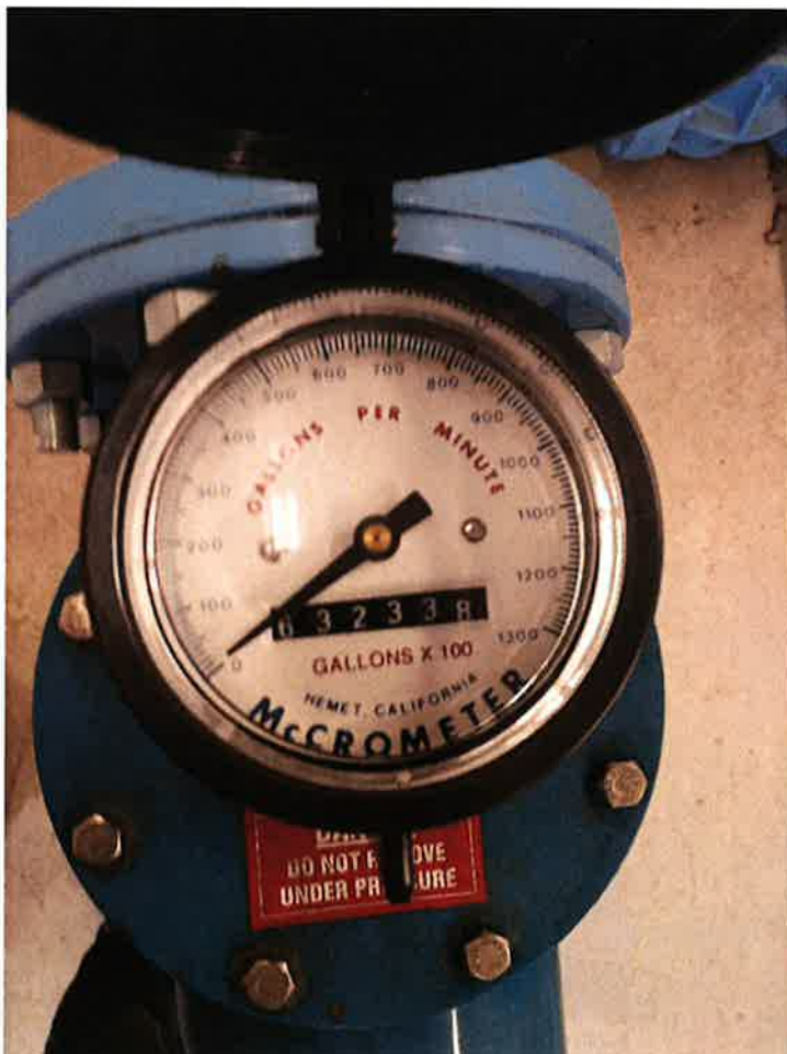
Figure 5 A flow meter installed at the older two wells.
