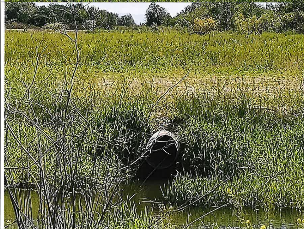
Corrugated pipe is placed every so often to drain flood water back into the dirt ditch and the Boise River.
