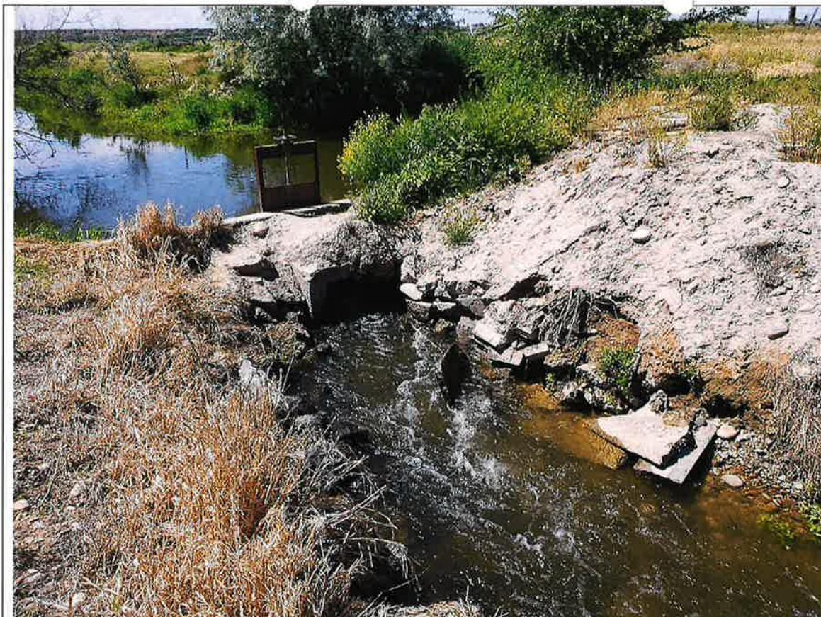
Point of Diversion from the Unnamed Drain. Slide gate was running about 40% capacity.
