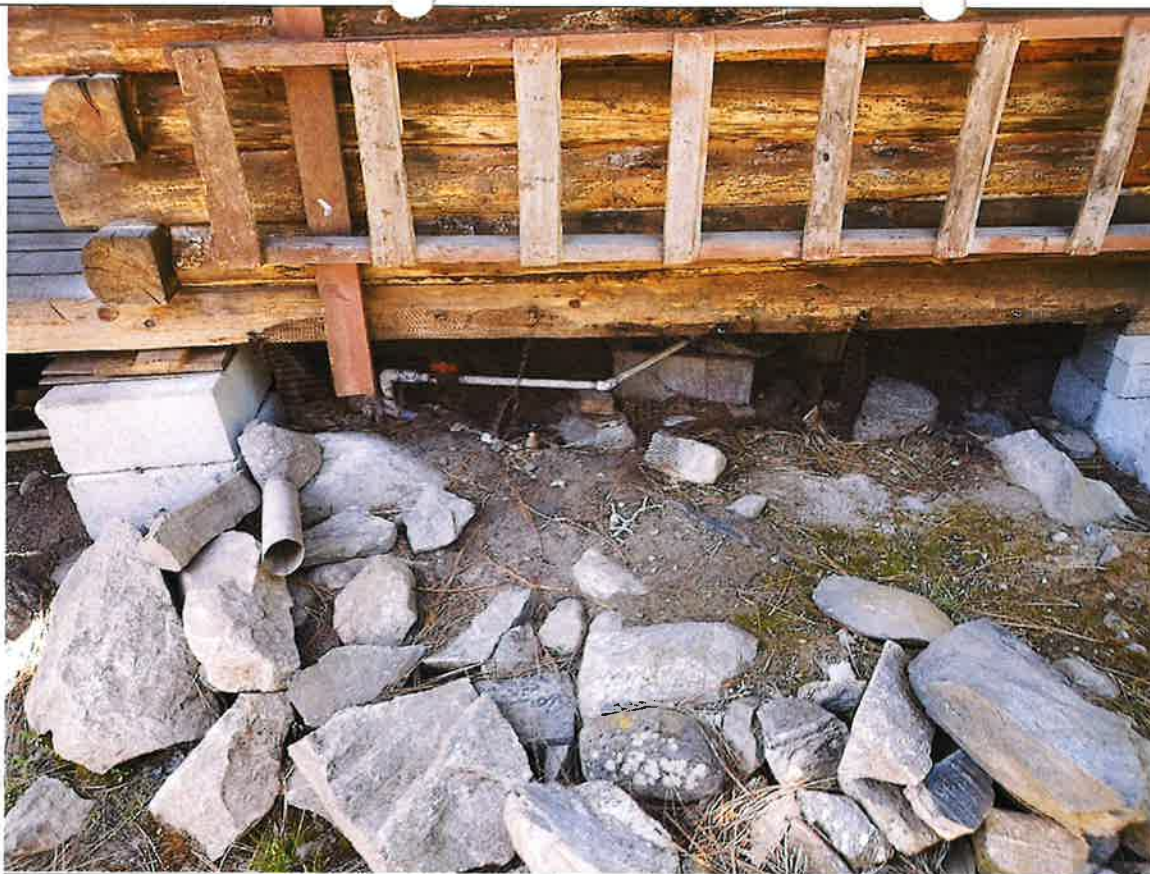
Water supply to the house.
