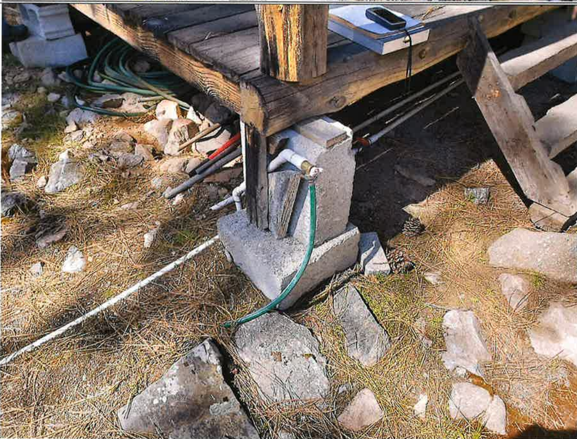
Hose bib below the front patio.
