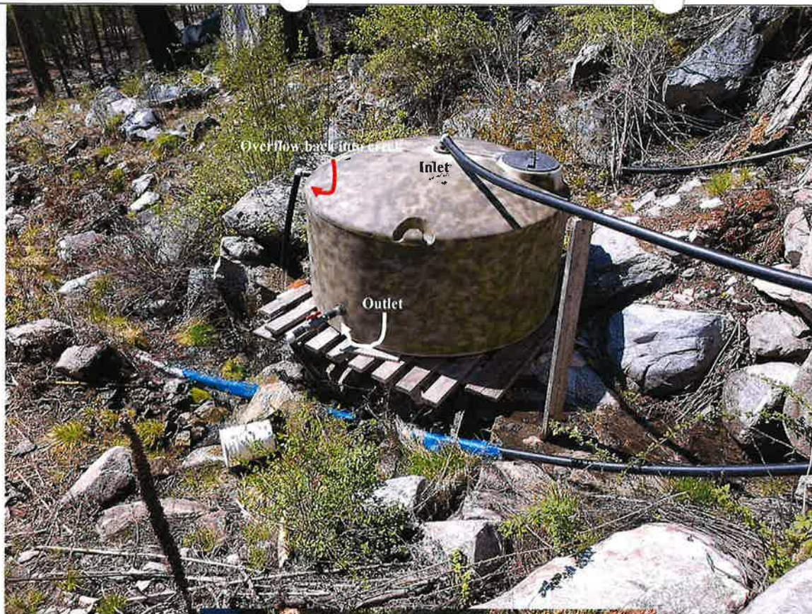
1,000 gallon tank that holds water for the two cabins.
