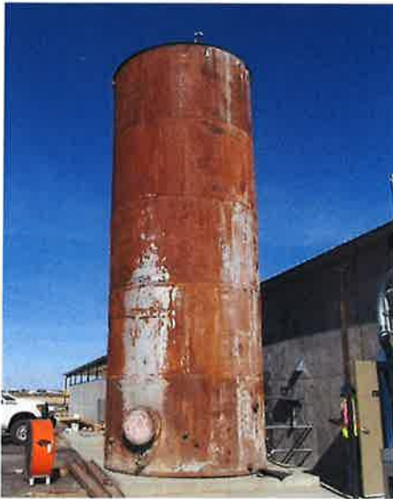
16,000 gallon storage tank for dairy #2
