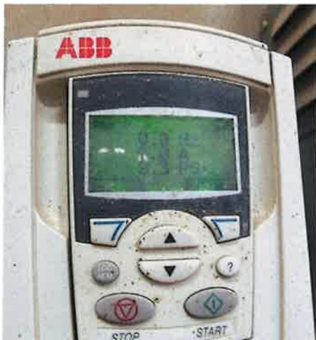
South Well variable speed box (9.3 psi)
