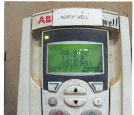
North Well variable speed box (55.8 psi)
