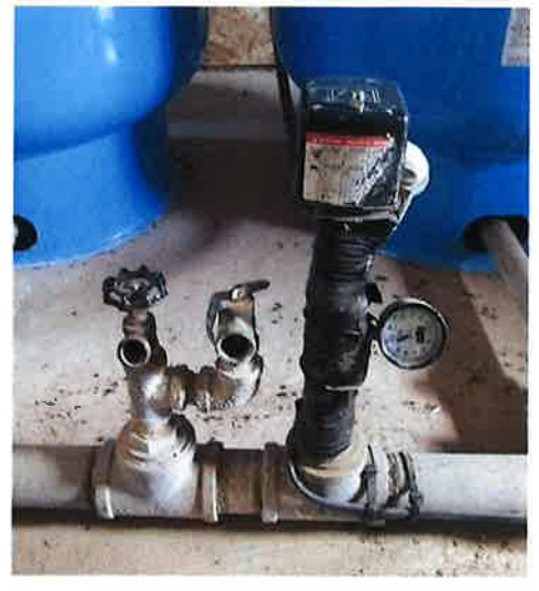
Pressure tanks for dairy #2 well (45 psi)
