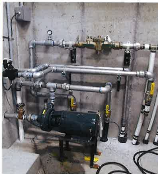
water distribution for dairy #2
