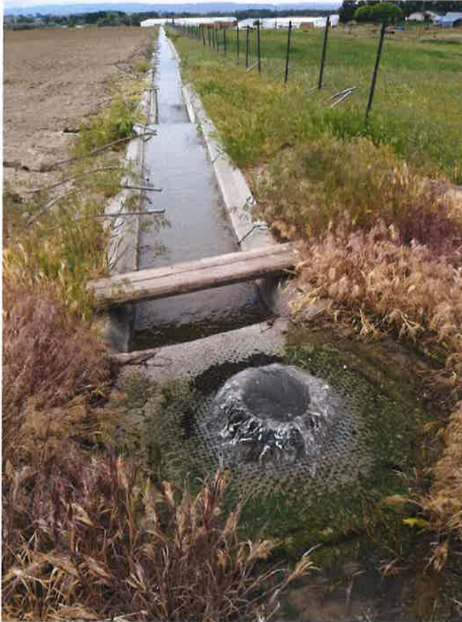
Figure 5 The second discharge pt. The water shown here is Farmers Coop water. There is no separate pipe from the pump at this location. The owner says that the pump is tied into the Farmers Coop system.
