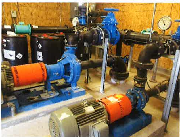
Overall view inside booster pump station
