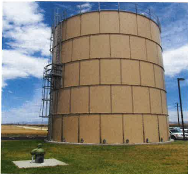
40' high 252,866 gallon water storage tank (wellhead visible on bottom left side)
