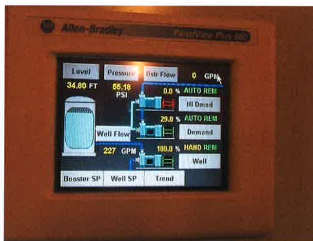
Booster pumps at 100% capacity (227 gpm)
