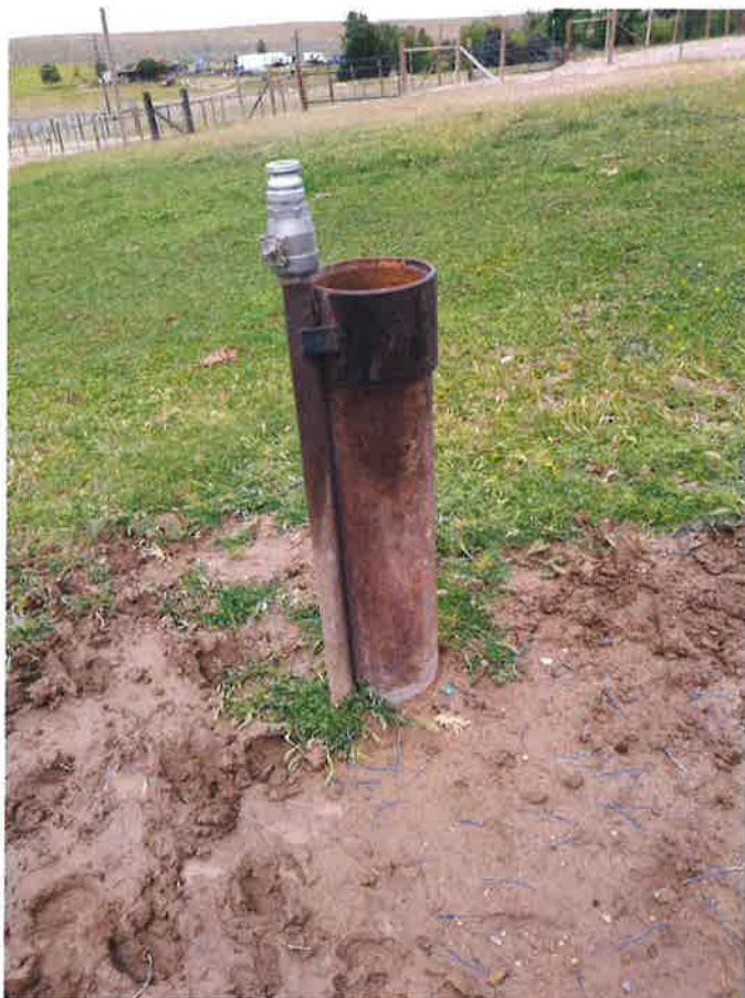
Figure 3 2" risers come off of the mainline and feed water to impact sprinklers. The risers are welded to old well casing for stability.
